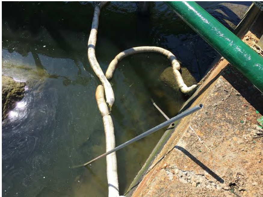
Figure 26: Sorbent booms installed adjacent to seawall.
