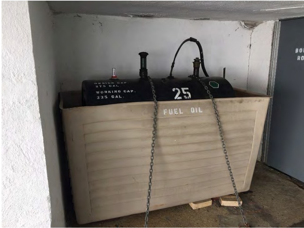
Figure 23: View of 275-gallon fuel oil ASY for heating system on western side of the office building.
