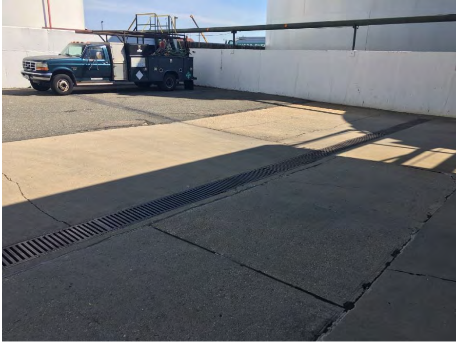
Figure 9: Trench drain located in the central portion of the site near the filling area.
