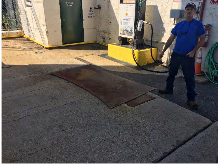
Figure 5: Oil water separator underneath steel plate with diesel fuel pump in background.
