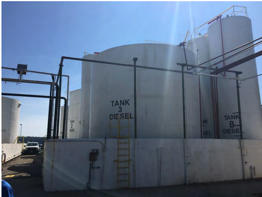
Figure 8: ASTs located on eastern portion of the property.
