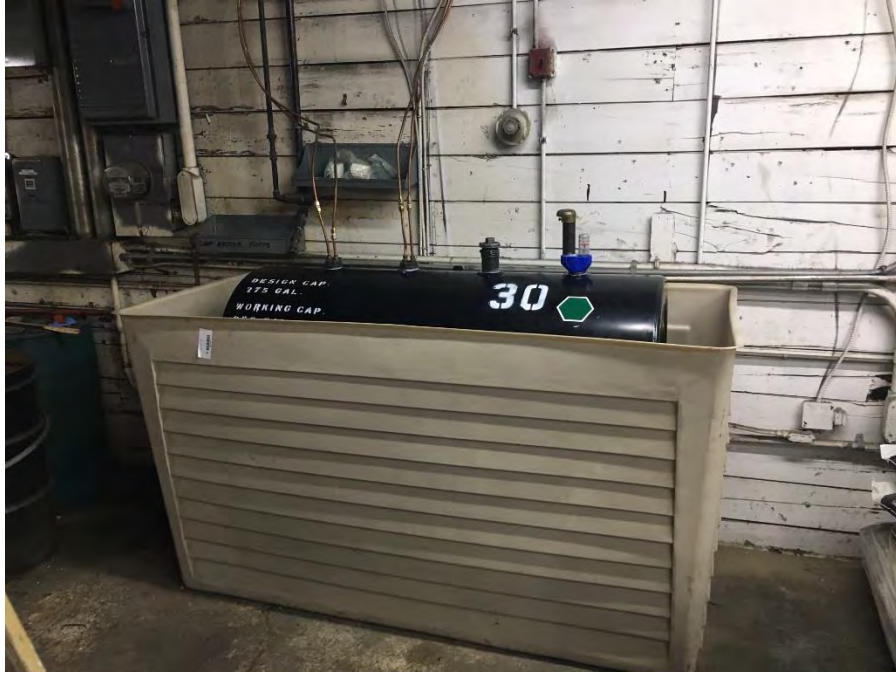
Figure 15: 275-gallon Fuel-Oil AST for garage building heating system.
