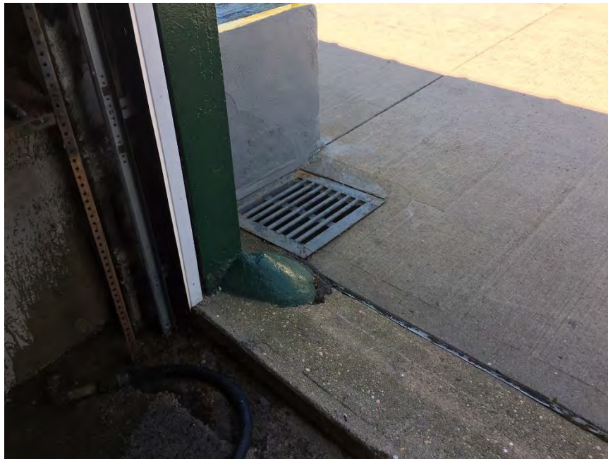
Figure 4: Catch basin where sump water is discharged to.
