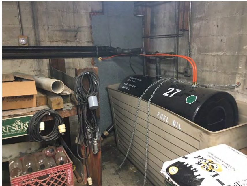
Figure 2: 275- gallon fuel oil AST located in eastern portion of office building.
