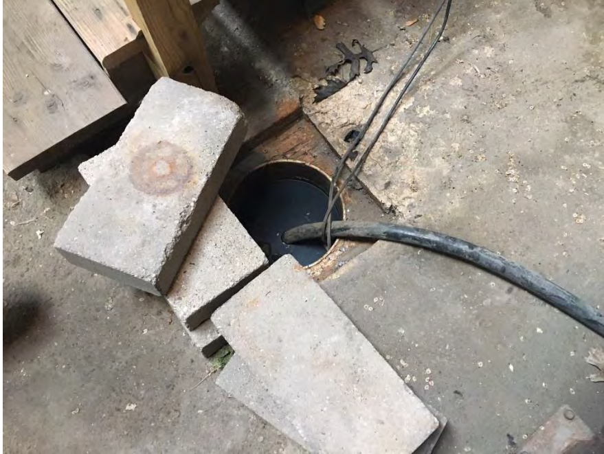
Figure 3: Sump located in office building maintenance area
