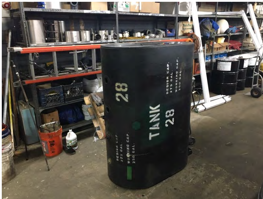
Figure 18: Out of service fuel oil AST staged in garage.
