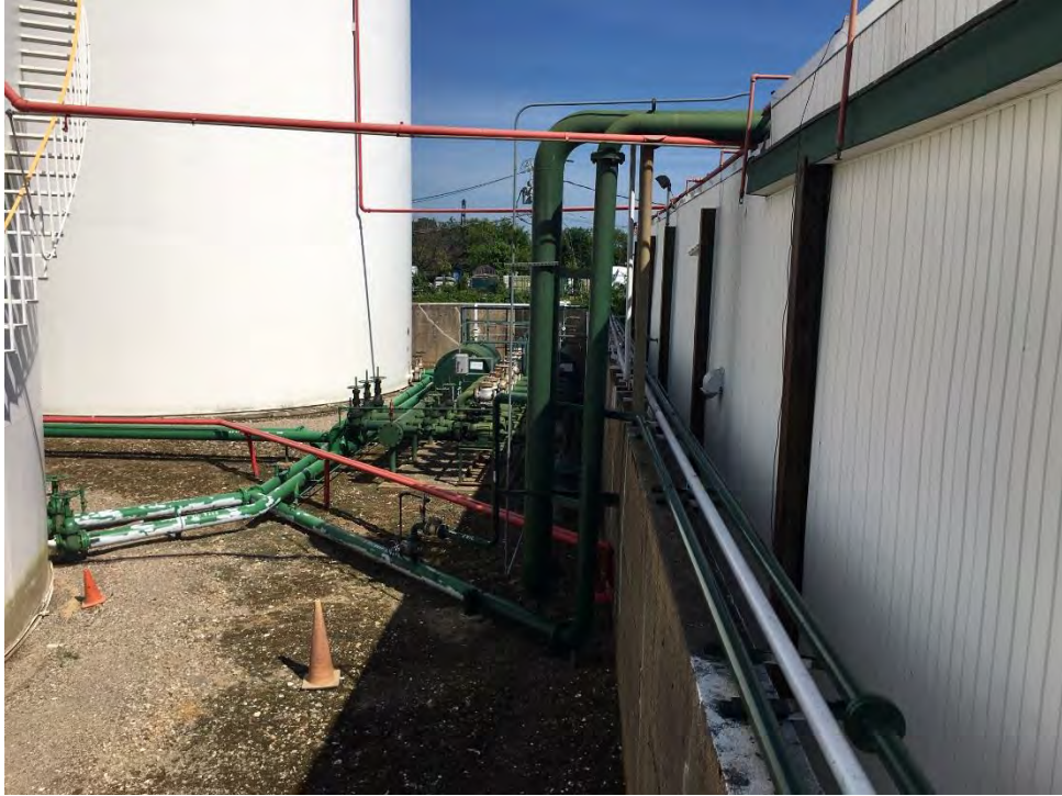
Figure 21: Interior of the western containment area with the three chemical ASTs in the background.
