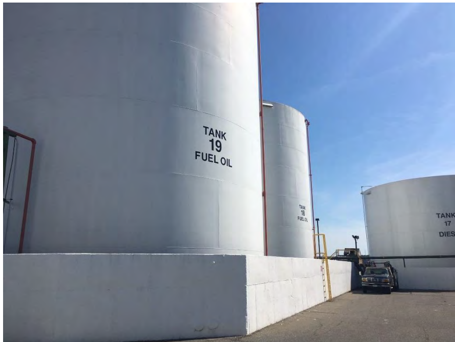
Figure 12: View of fuel-oil ASTs
