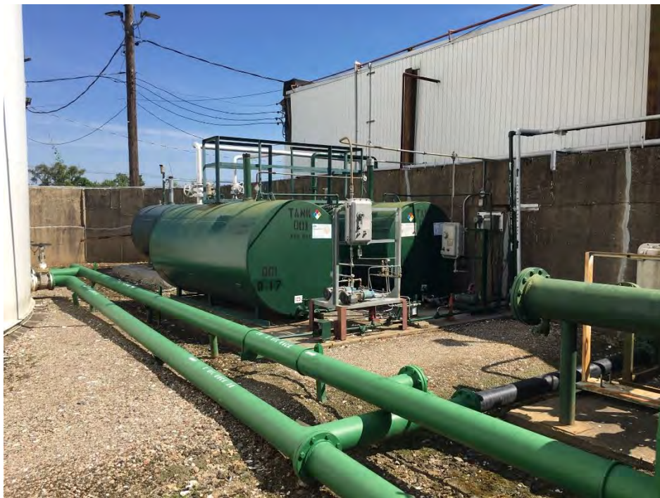
Figure 22: Image of chemical ASTs within the western containment area.
