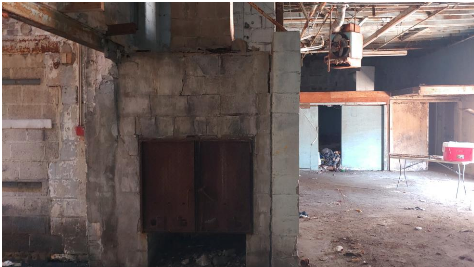
23. View of incinerator located in the rear southwest corner of building
