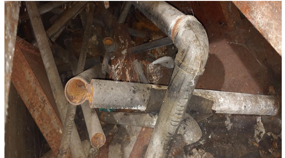
4. Jumble of piping and possible drum or tank in Sump in basement
