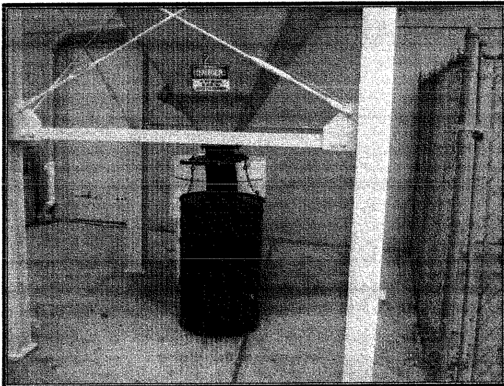
Photograph 8: View of dust collector at 303 Prospect Street
