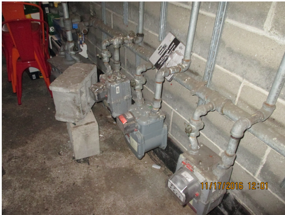
Gas services meters and piping.
