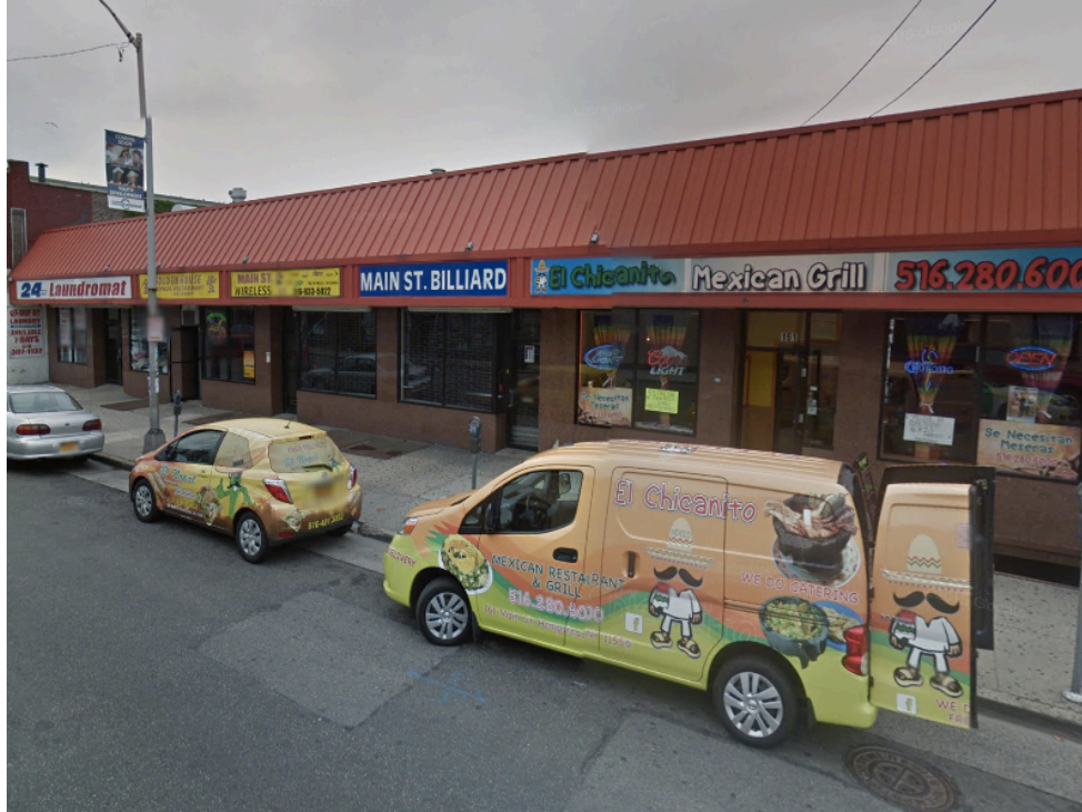
Commercial Building – Main Street Exterior roof flashings contain asbestos.
