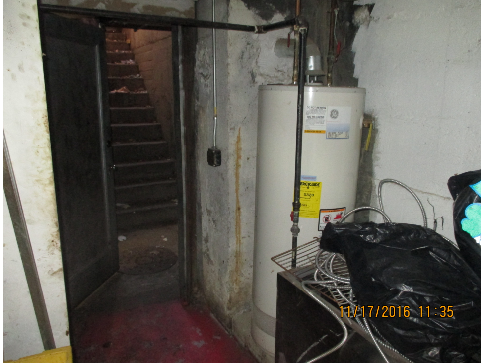
Typical - Domestic Hot Water Heater No asbestos materials identified.
