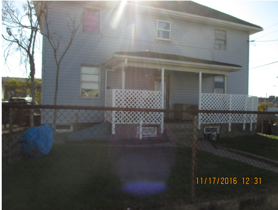
122 Bedell Street – occupied. Limited access, additional inspection required.
