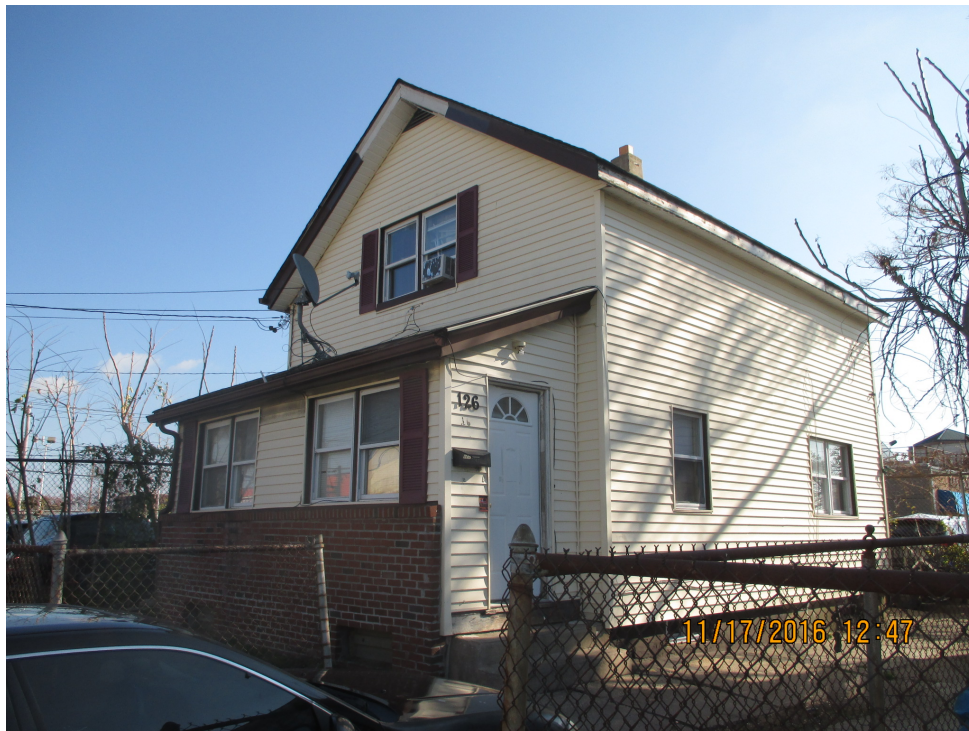
126 Bedell Street – occupied. Limited access, additional inspection required. Transite asbestos shingles are under the vinyl siding.
