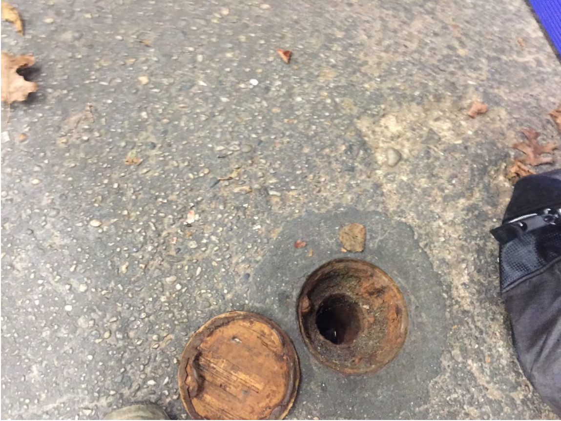
Photograph No. 13: Typical interior small diameter drain located in the golf bag room.
