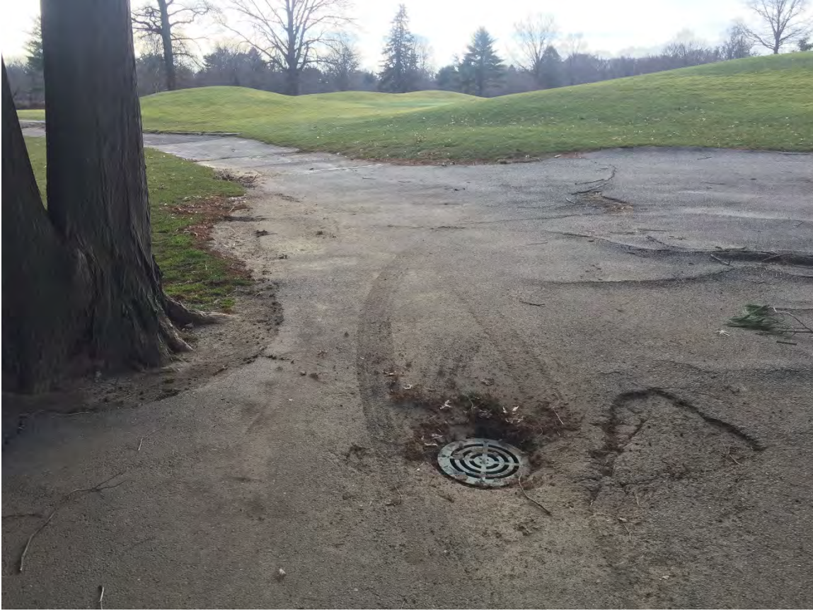
Photograph No. 15: Typical makeshift drywell located on the cart paths and golf course.
