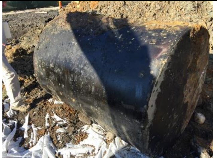
PHOTO 4: Detail shot of pin-holes observed following removal of UST
