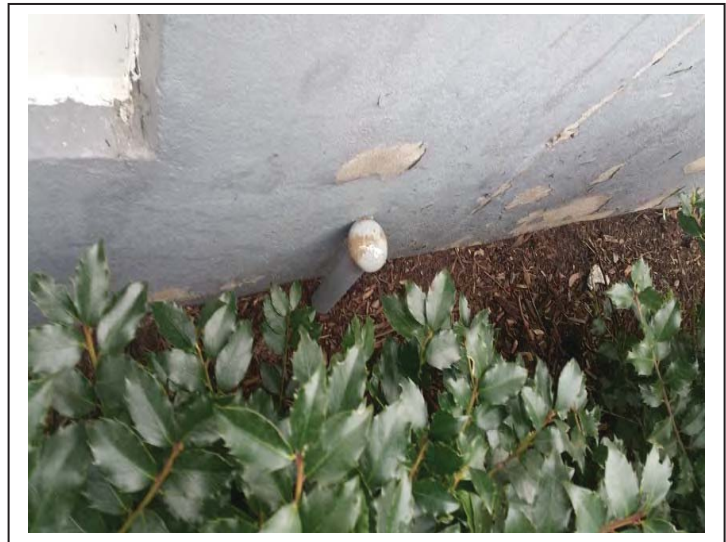
VENT FOR UST
