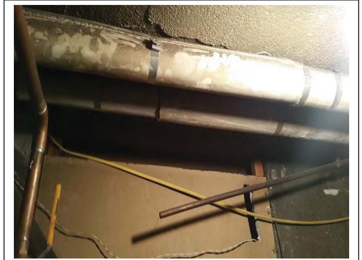
ACM ON OVERHEAD PIPE
