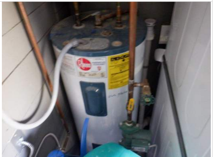
14. Hot water heater
