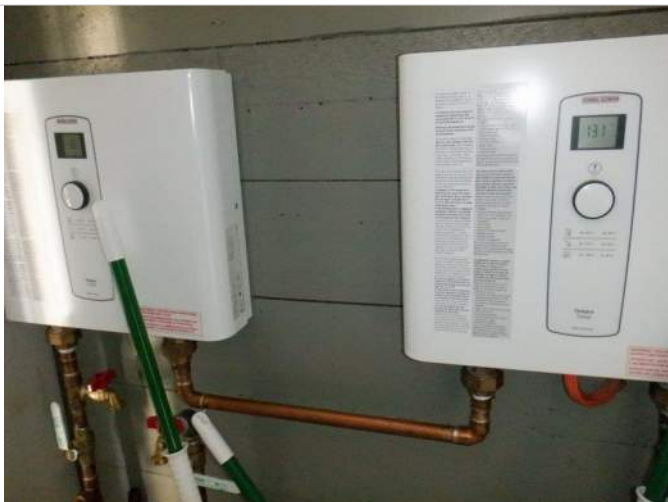
13. Tankless hot water heaters
