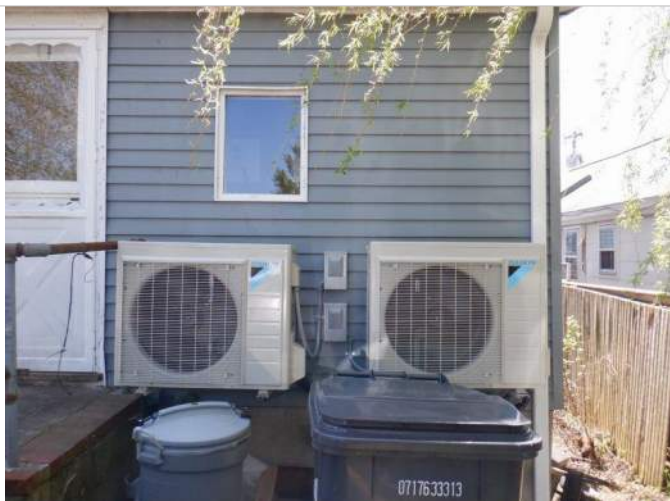
9. AC units behind building
