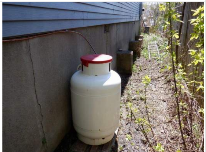
10. Propane tank to west of building
