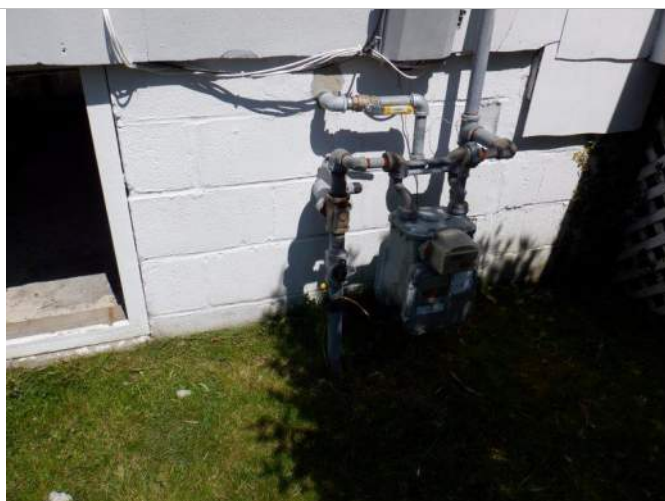
16. Gas meter for main building
