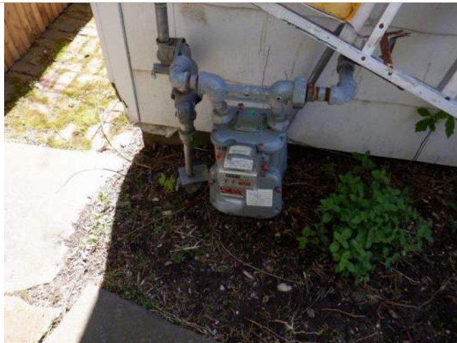
12. Gas meter for apartment building
