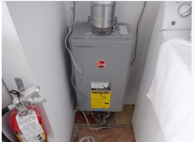
20. Heating unit for main building
