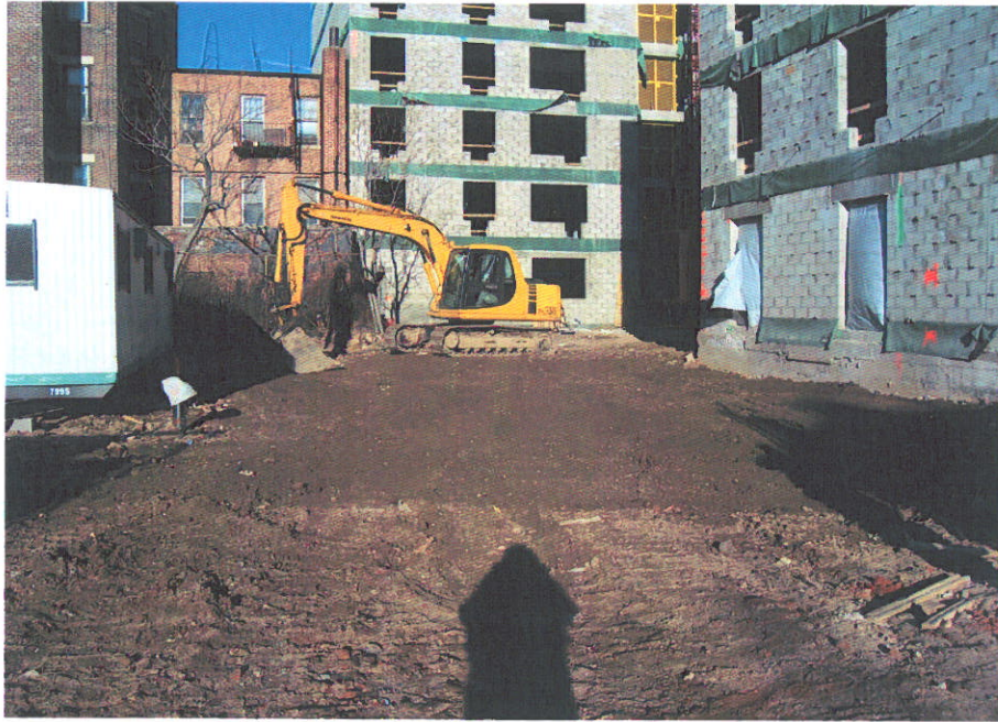
23. Clean fill being spread on top of catch basin in parking area (taken from E. 160 th Street)
