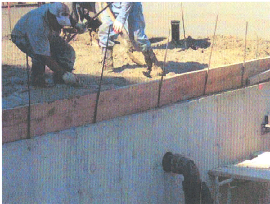
28. Slab on grade installation in progress adjacent to cellar along column line 4
