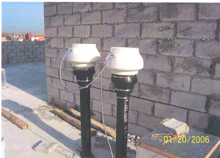
26. FR-250 fans, atop portion of structure adjacent to E. 161 st Street
