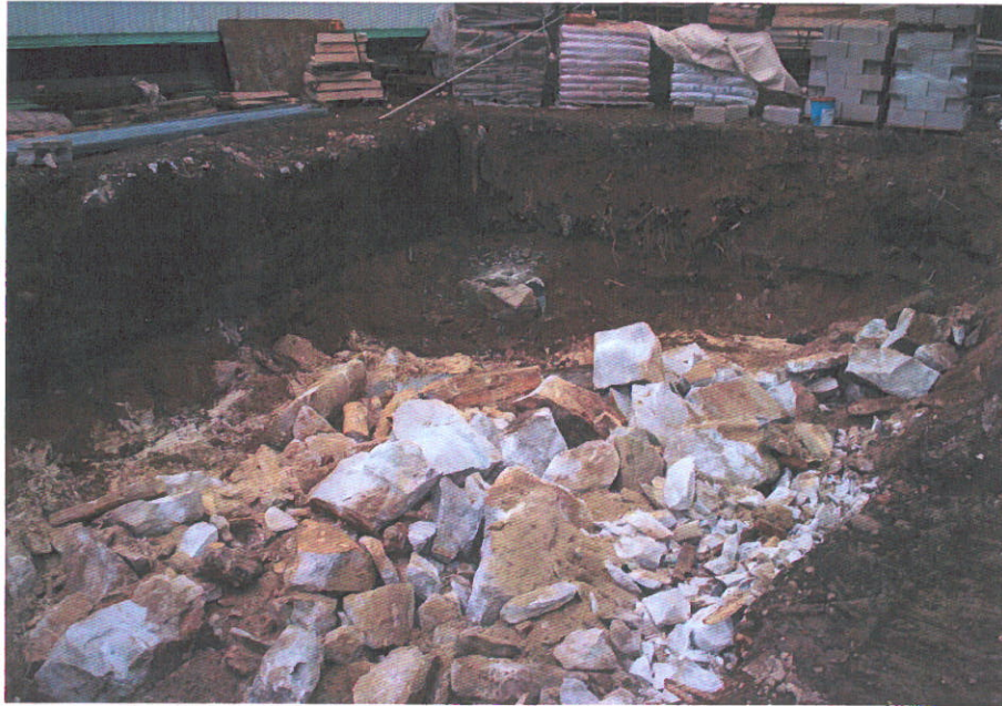
21. Broken bedrock in catch basin (in parking area)
