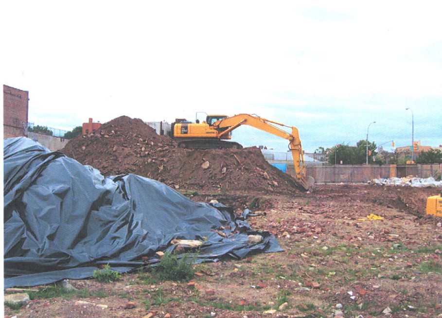
10. Covered, pesticide-contaminated soil (foreground), and stockpiled material from the basement area (background), looking northeast
