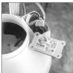
Romex wiring – Top View
