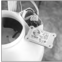
Romex wiring – Top View
