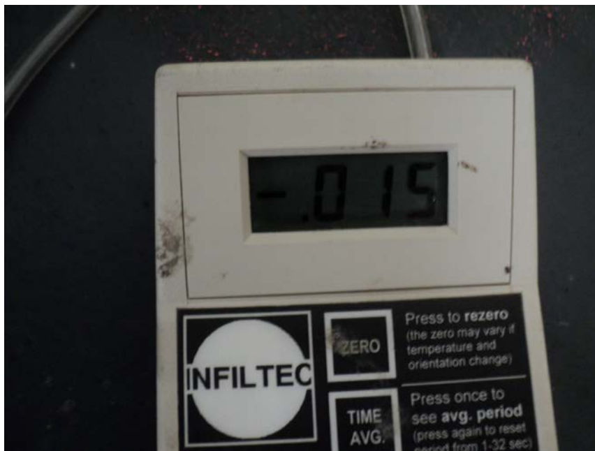
10. Vacuum reading at VEMP-2 on December 2, 2016.
