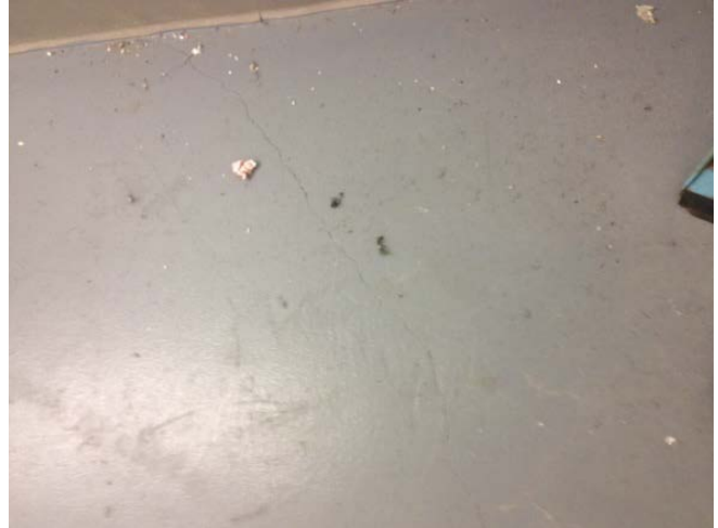
Photo 8: View of typical bare floor in Room C59.
