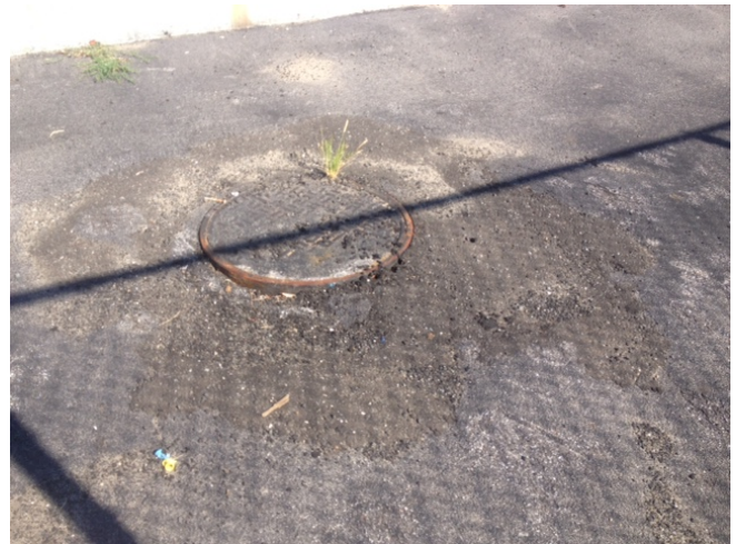
Photo 10: View of repairs made to the manhole by the East Access Drive.
