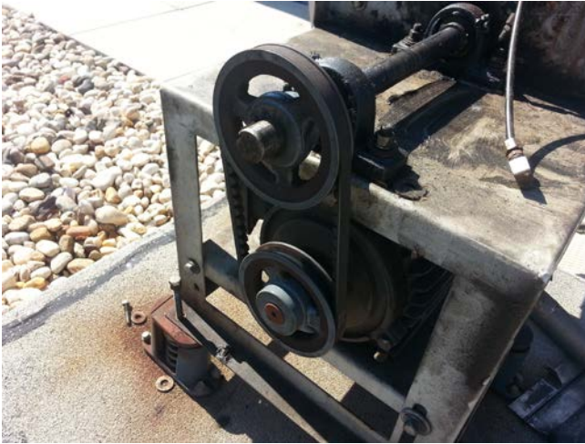
Photo 7: View of typical SSDS fan belt and assembly (EF-6).
