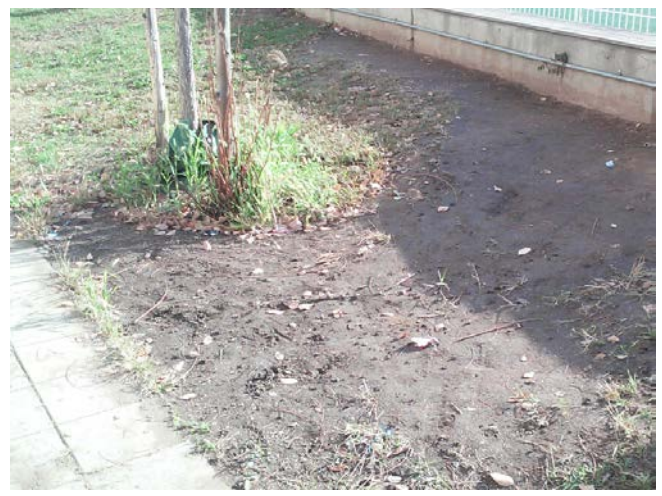
Photo 12: View of repairs made to the minor depression (4'x 2'x 4") at the east end of the artificial turf.
