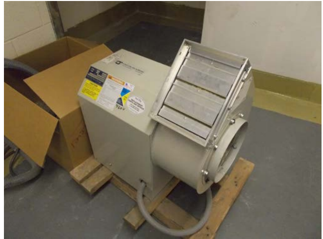
Photo 2: View of spare SSDS fan unit (EF-7) in Room B80.
