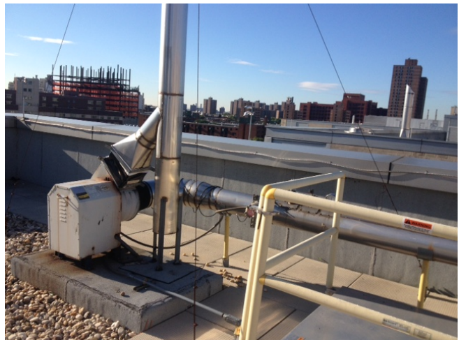
Photo 4: View of typical SSDS roof fan unit (EF-6).
