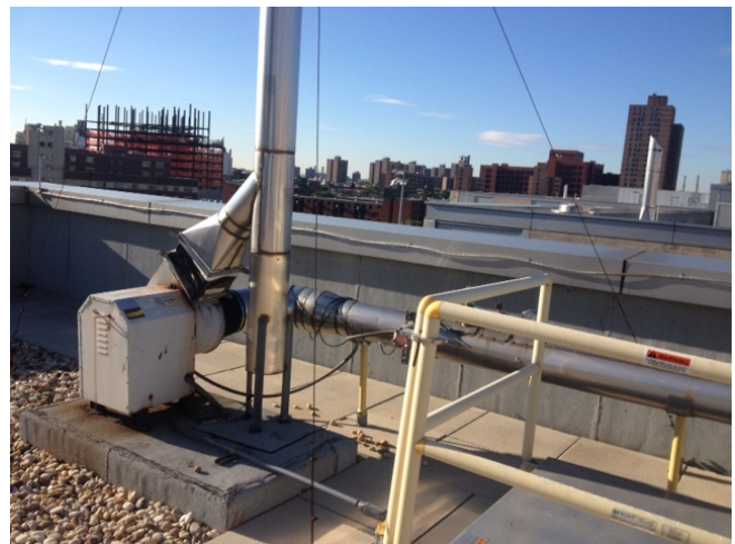
Photo 2: View of typical SSDS roof fan unit (EF-6).
