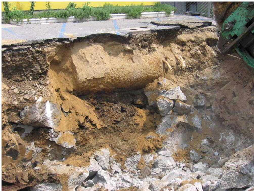
Tank4 – 550 gallon Fuel Oil UST
