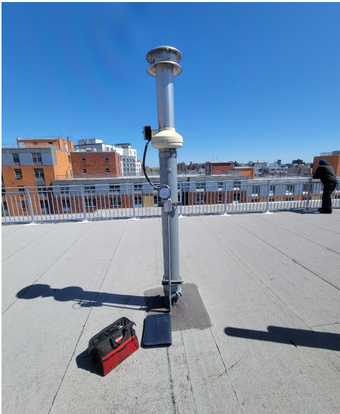
SSDS piping on the 8th floor.
