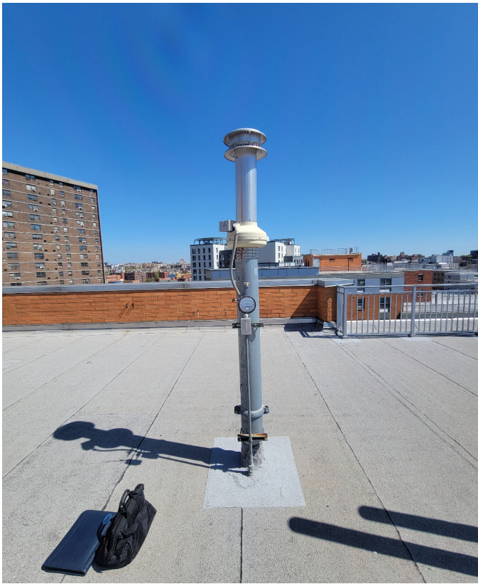
SSDS piping on 10th floor.
