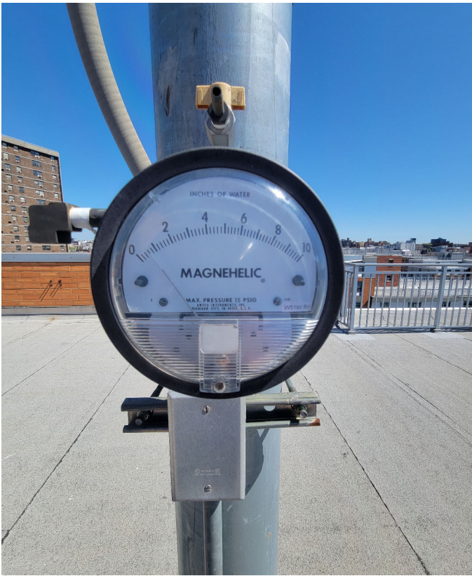
Vacuum gauge on 10th floor.
