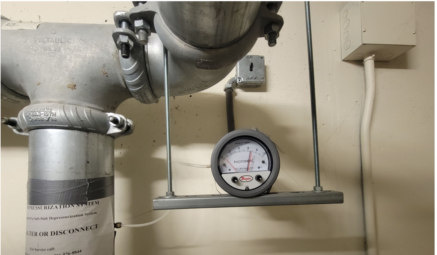
Vacuum gauge in Room C-07
