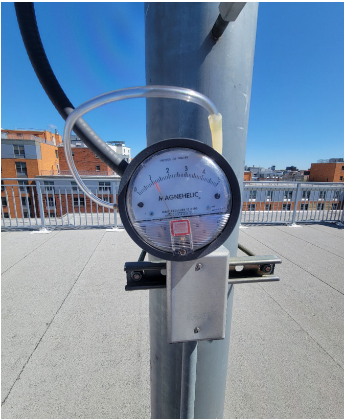
Vacuum gauge on the 8th floor.
