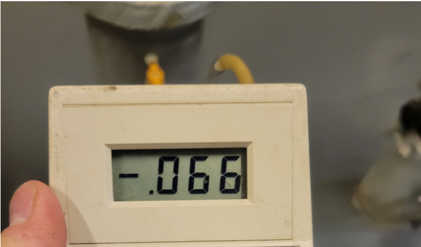
Vacuum at Riser C.
