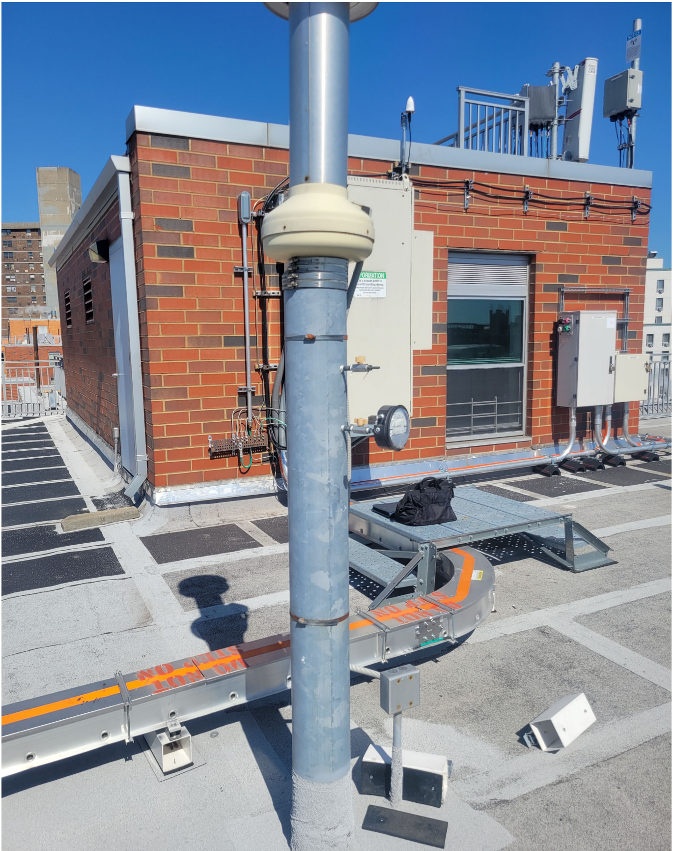
SSDS piping on the roof.
