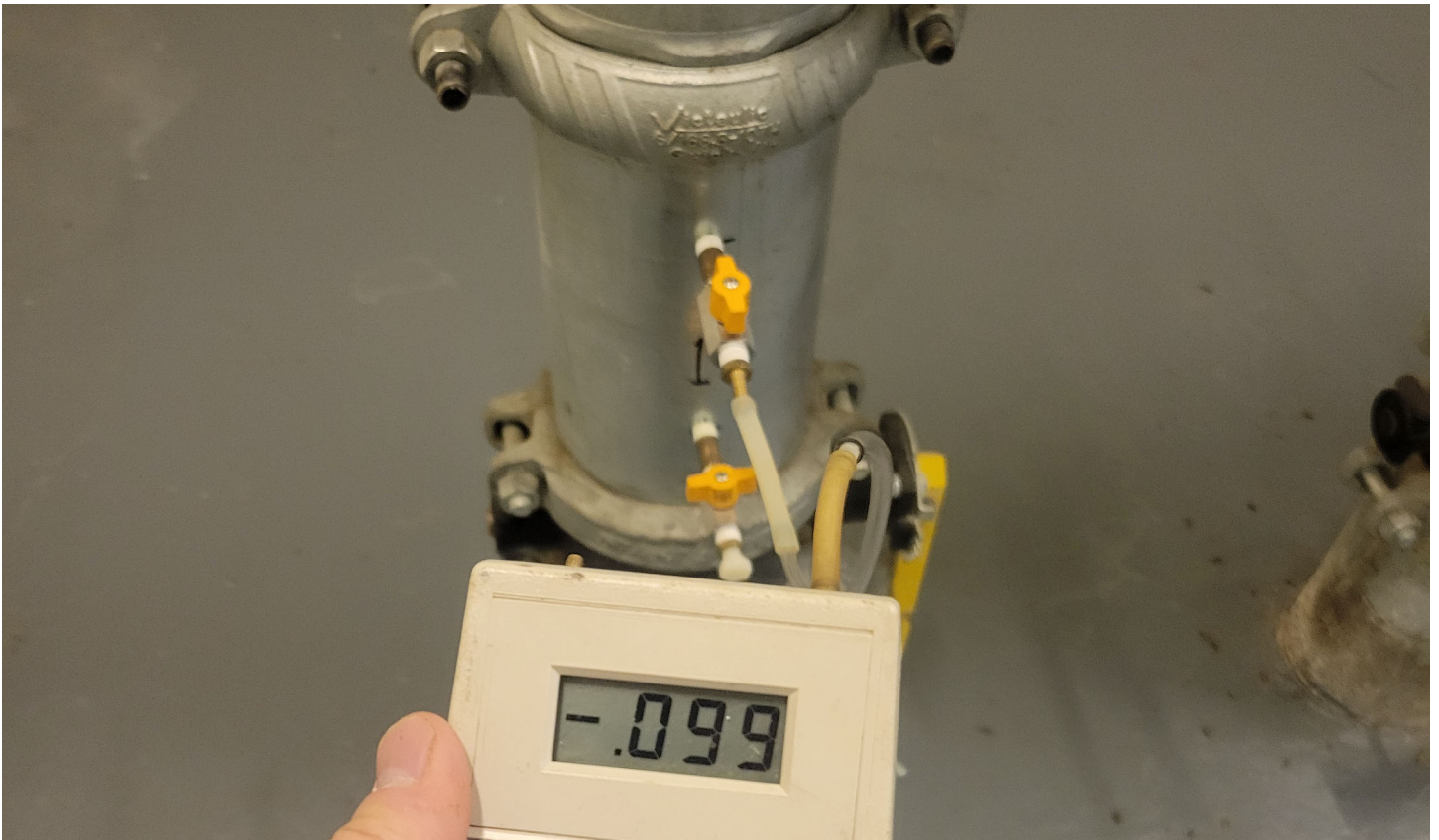
Vacuum at Riser A.
