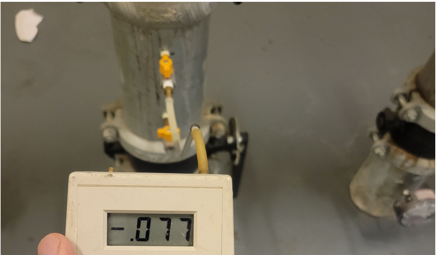
Vacuum at Riser B.
