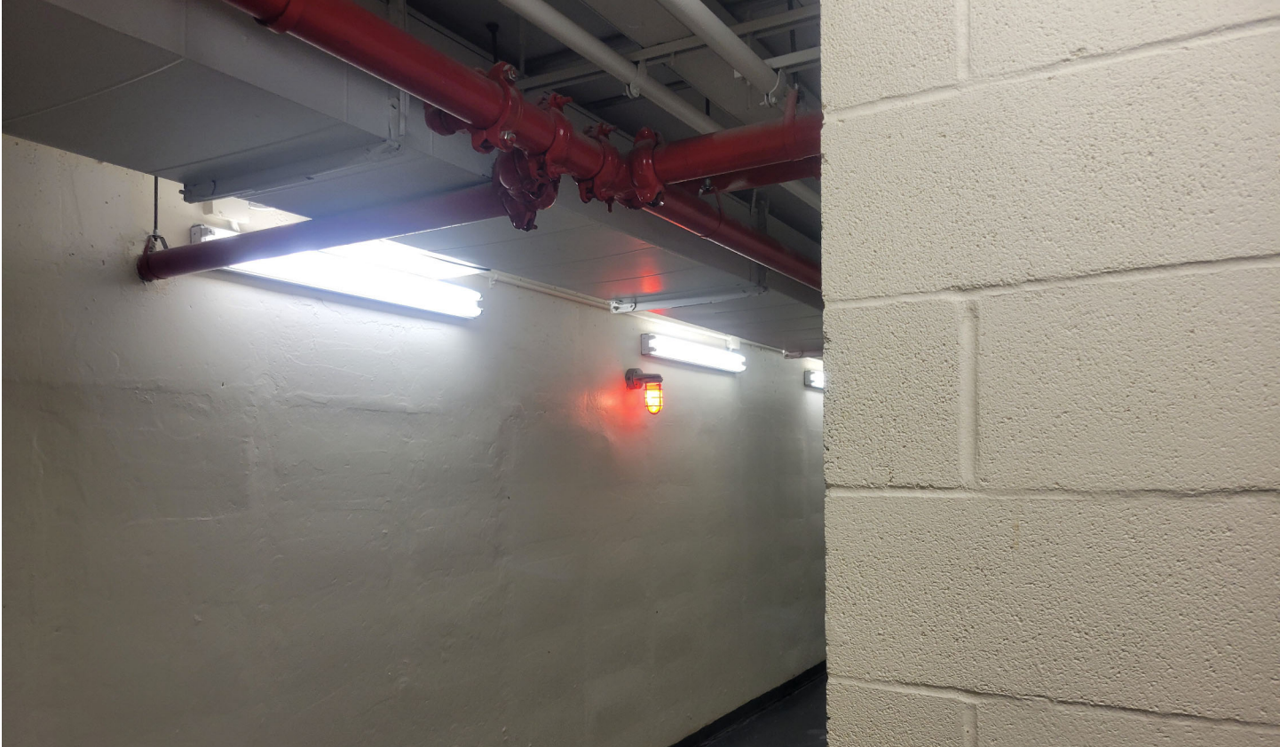
Testing the red light alarm.
