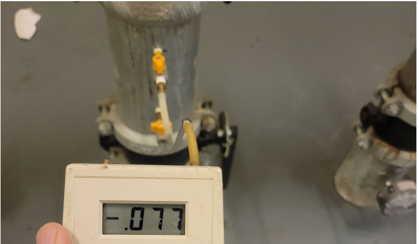
Vacuum at Riser B.
