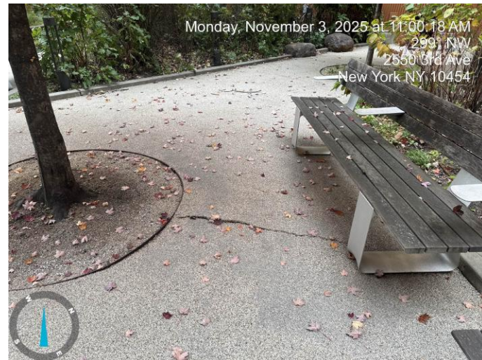
Photograph 4: Minor cracks in the pathways in the southern courtyard of the Tres Puentes West Building Site, facing west.
