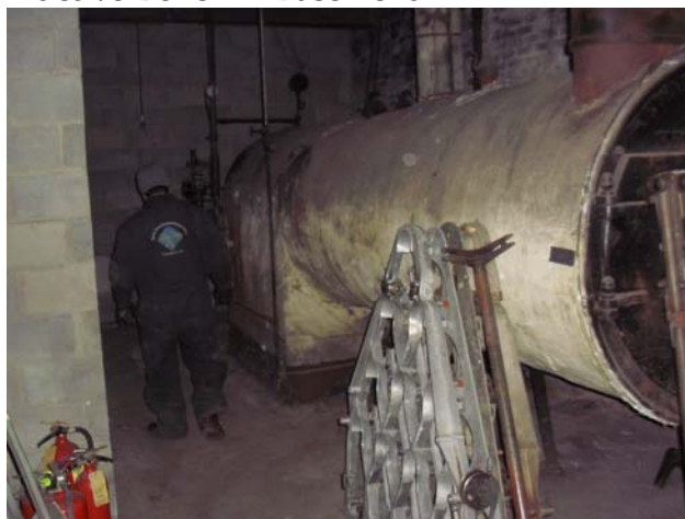
Inactive Boiler in Basement
