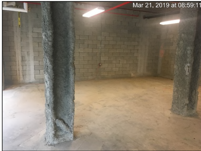
Photograph 13: Typical concrete slab on the ground level in the southwestern portion of the Site.
