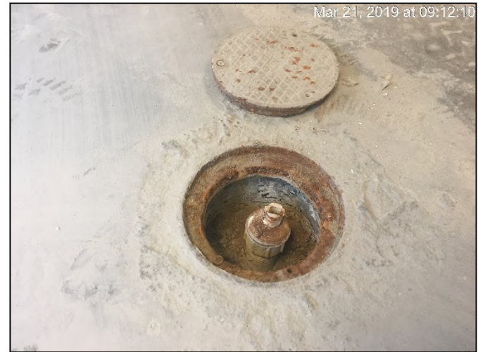
Photograph 14: Typical vapor monitoring point (MP-4).
