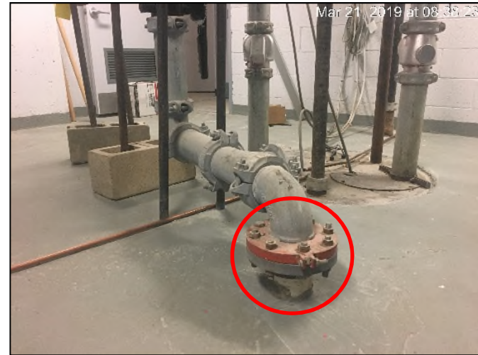
Photograph 10: Vertical riser VR-1A penetration in the telecommunications room in the partial cellar.
