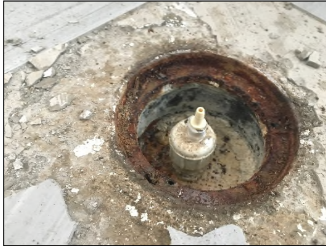
Photograph 1: Soil vapor monitoring point MP-5 in the partial cellar of the Site building.
