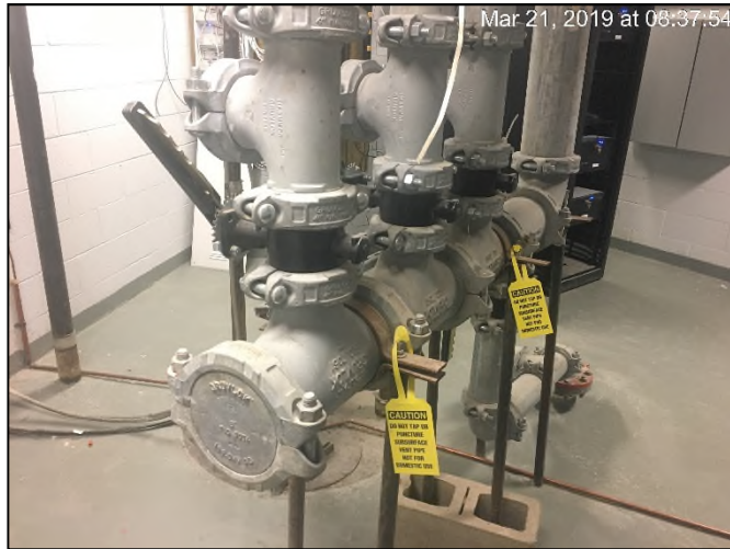
Photograph 9: Sub-slab depressurization system (SSDS) manifold in the telecommunications room in the partial cellar.
