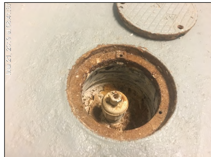
Photograph 12: Typical vapor monitoring point (MP-1).
