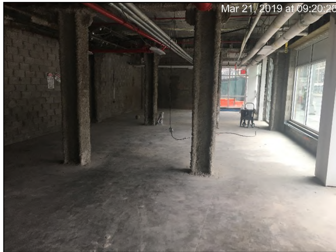
Photograph 15: Typical concrete slab on the ground level in the eastern portion of the Site.
