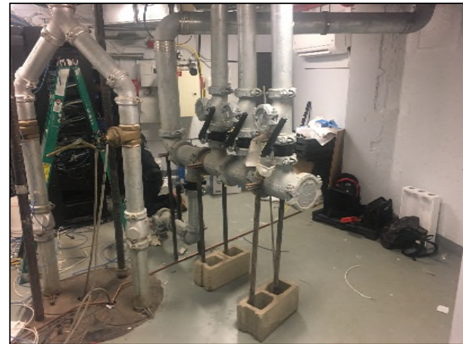
Photograph 8: Sub-slab depressurization system (SSDS) manifold in the telecommunications room of the partial cellar.
