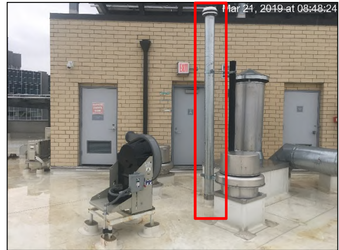
Photograph 16: SSDS exhaust stack with rain cap on the roof.
