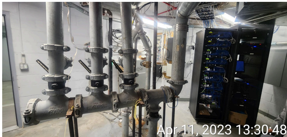
Photograph 14: Sub-slab depressurization system (SSDS) manifold in the cellar-level telecommunications room.
