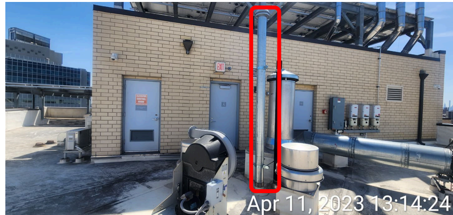
Photograph 15: SSDS exhaust stack with rain cap on the 12 th floor roof.
