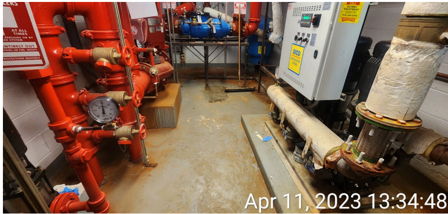
Photograph 9: Typical partial cellar slab in the cellar-level water meter fire pump room.
