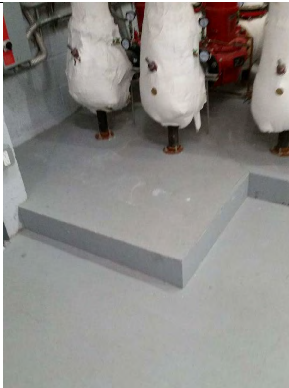
Photograph: 22 Equipment pad showing crack
