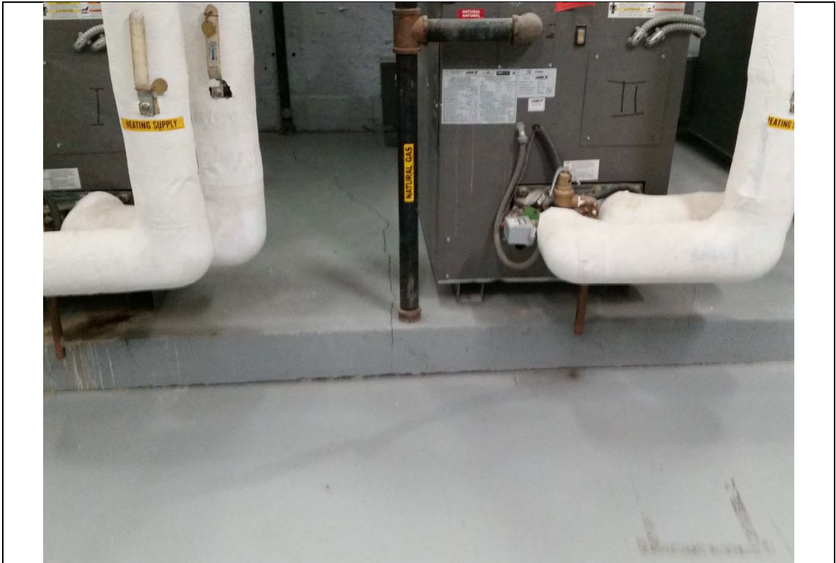
Photograph: 23 Equipment pad showing crack
