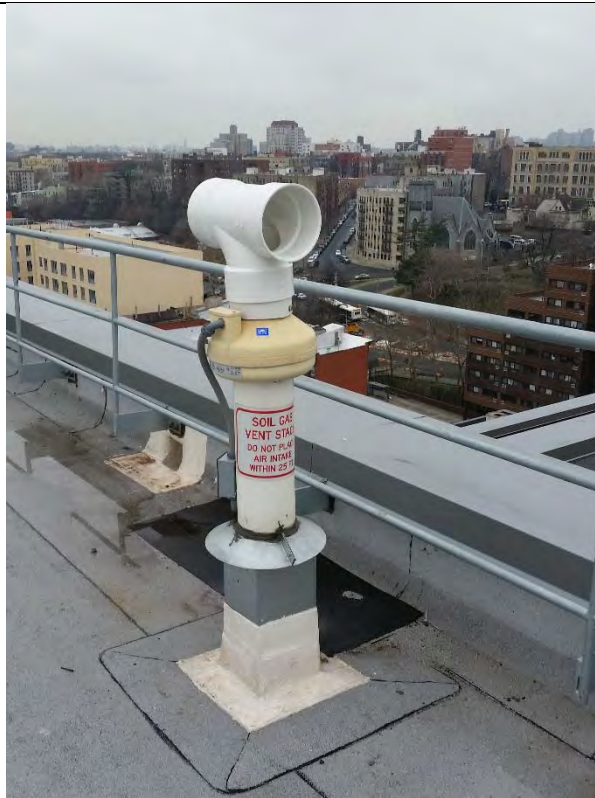
Photograph: 30 Exhaust Stack
