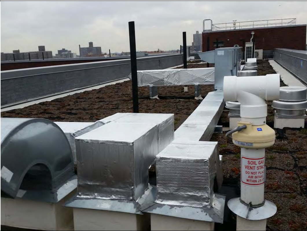
Photograph: 31 Exhaust Stack
