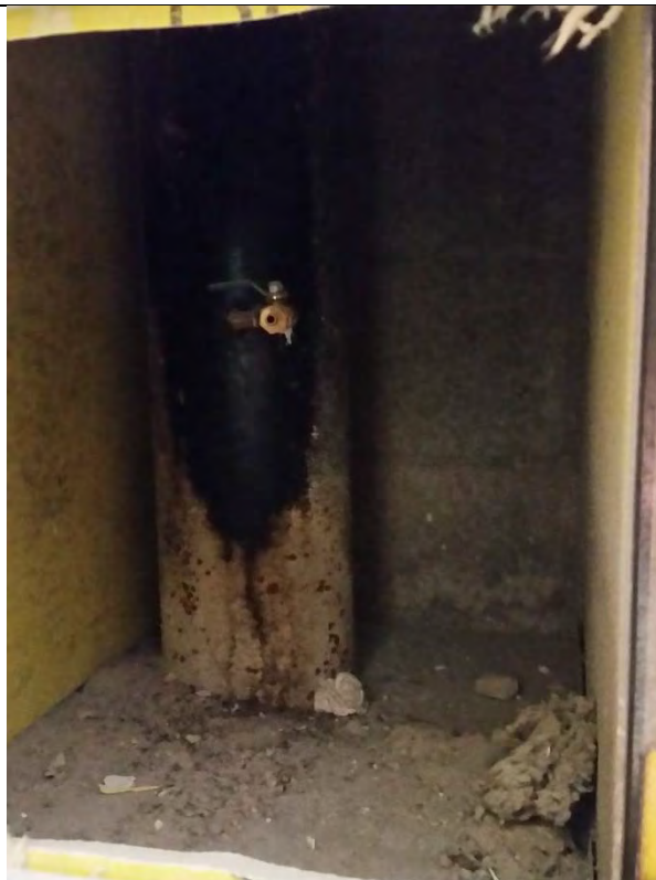
Photograph: 10 SP-01 access in electric/telecom room
