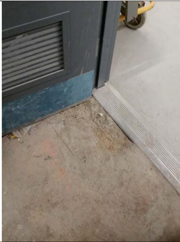
Photograph: 29 Damaged slab in doorway
