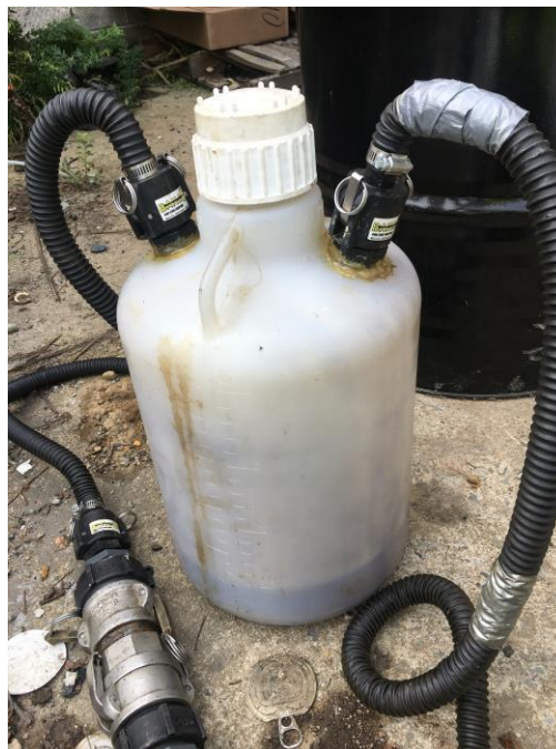
Photo 2: Knockout pot used to fluid recovery flow rate measurements
