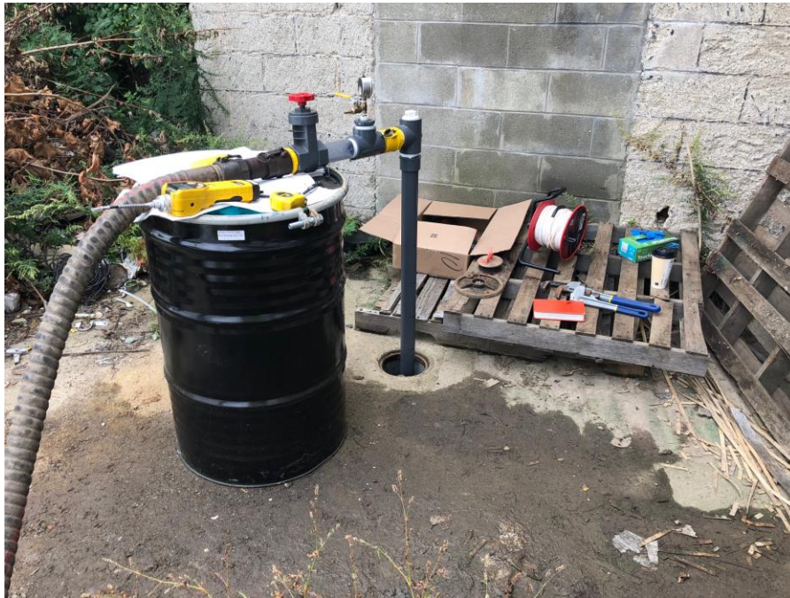
Photo 1: Wellhead assembly on stinger drop tube
