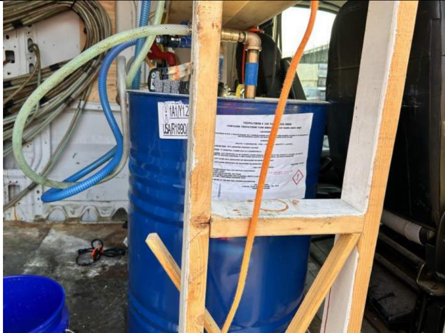
Photo 1: View of Tripolymer® 105 Tank Media Resin in container inside Endeavour's support vehicle (facing north).
