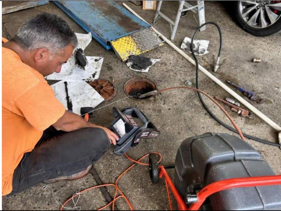
Photo 3: View XRAY field personnel preparing for a camera inspection of the UST interior.
