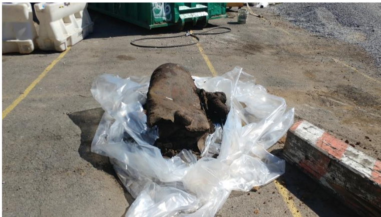
Photograph 3. A 100-gallon tank and piping were discovered in Grid A2, and were placed on plastic for future cleaning and disposal.
