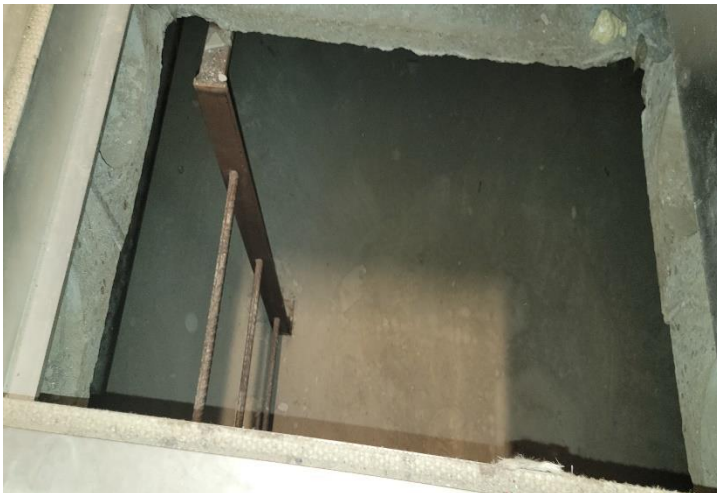
Photograph 3: A crawl space access hatch and a portion of the crawl space slab located within the northeastern section of the Track 4 portion of the Site.
