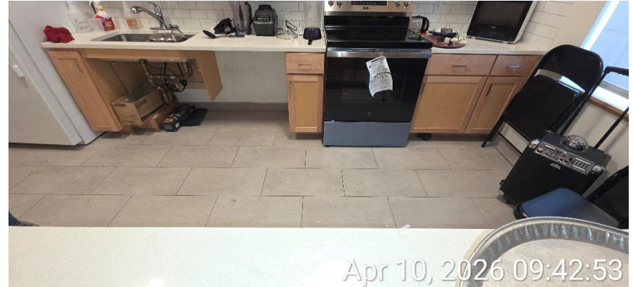
Photograph 2: The kitchen within the residential unit on the ground floor, view facing south.
