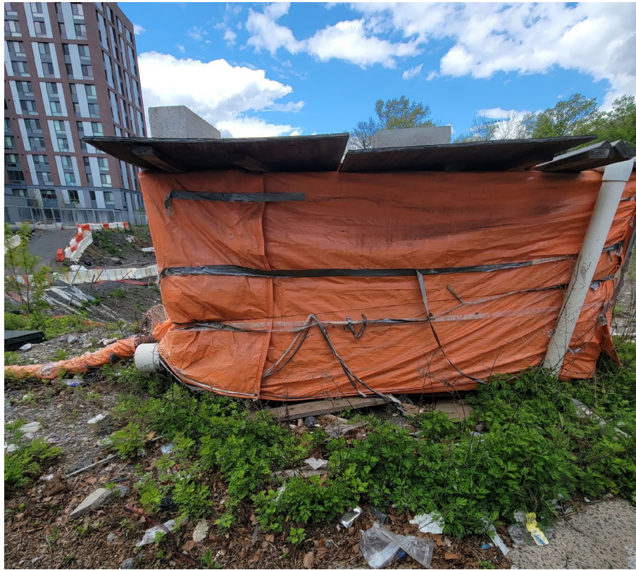
Photograph 1: Facing North, 300-gallon setting tank for operating onsite dewatering system.
