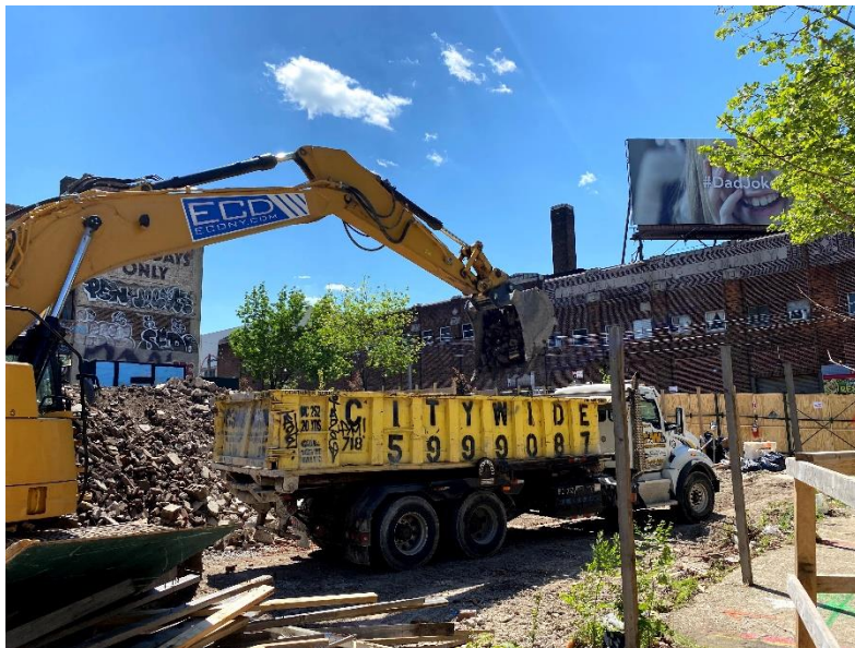
Photo 4: View of ECD NY Inc. (ECD) loading a truck with construction and demolition (C&D) material for off-site disposal, facing southeast. Taken on 05/11/2021
