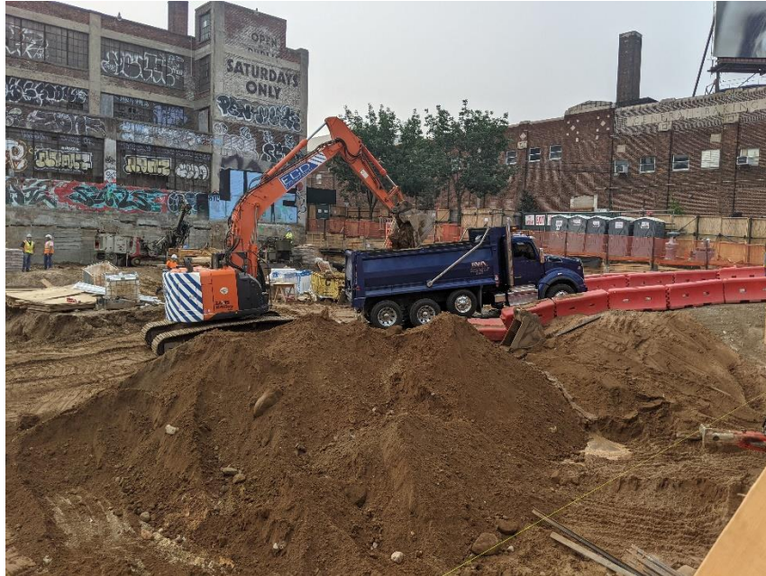
Photo 11: View of ECD loading a truck with non-hazardous soil for off-site disposal, facing southeast. Taken on 07/20/2021
