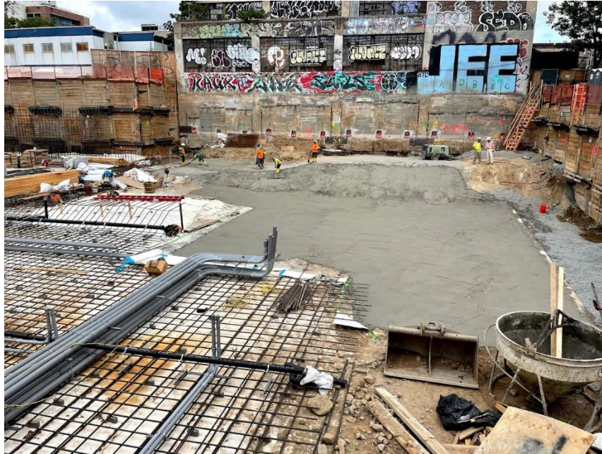
Photo 15: View of concrete rat slab poured in the central part of the site, facing east. Taken on 08/18/2021
