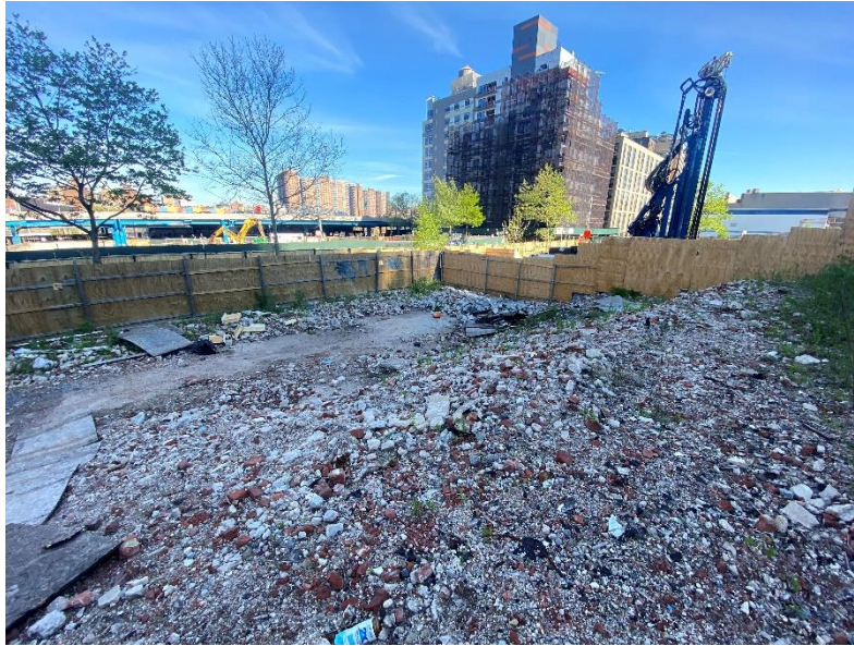
Photo 3: View of site prior to mobilization for excavation activities, facing northeast. Taken on 05/07/2021
