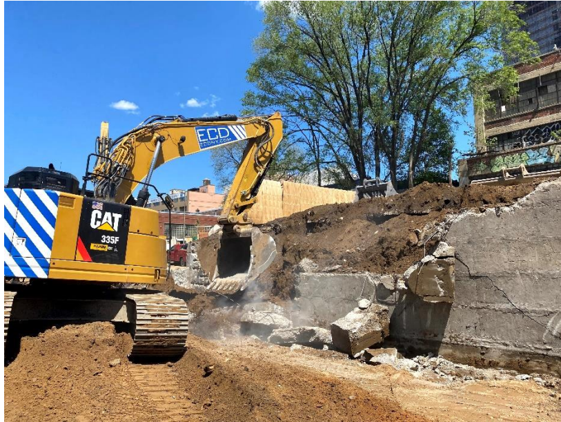
Photo 5: View of ECD breaking a foundation wall in the central part of the site, facing northeast. Taken on 05/14/2021
