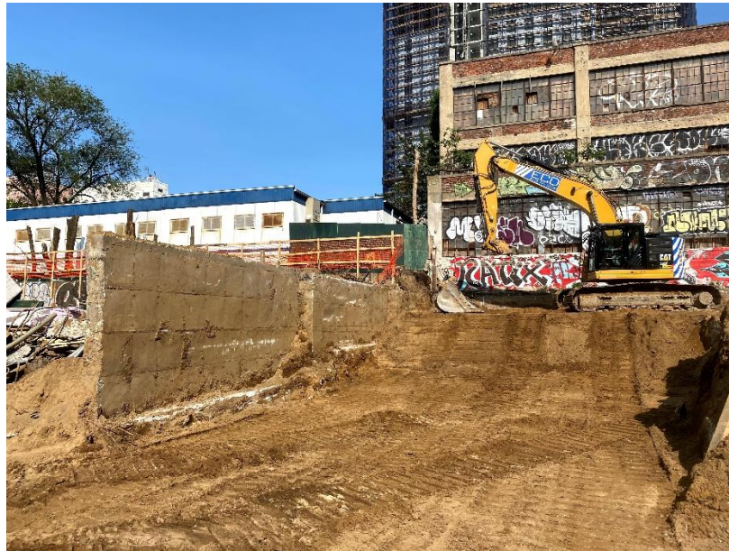
Photo 7: View of ECD excavating the northeastern part of the site, facing east. Taken on 05/19/2021
