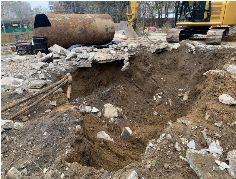
Photo 1: View of 3,000-gallon UST and excavated UST grave, facing northwest. Taken on 12/09/2020
