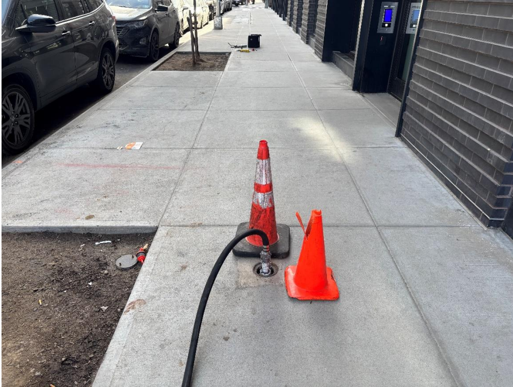
Photo 1: Injection housing and fittings connected to OMW-01.
