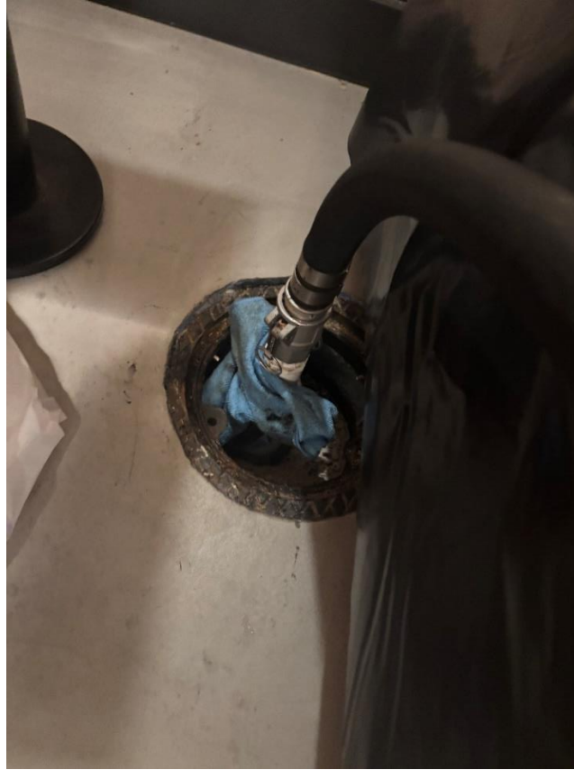
Photo 1: Injection housing and fittings connected to RMW14.
