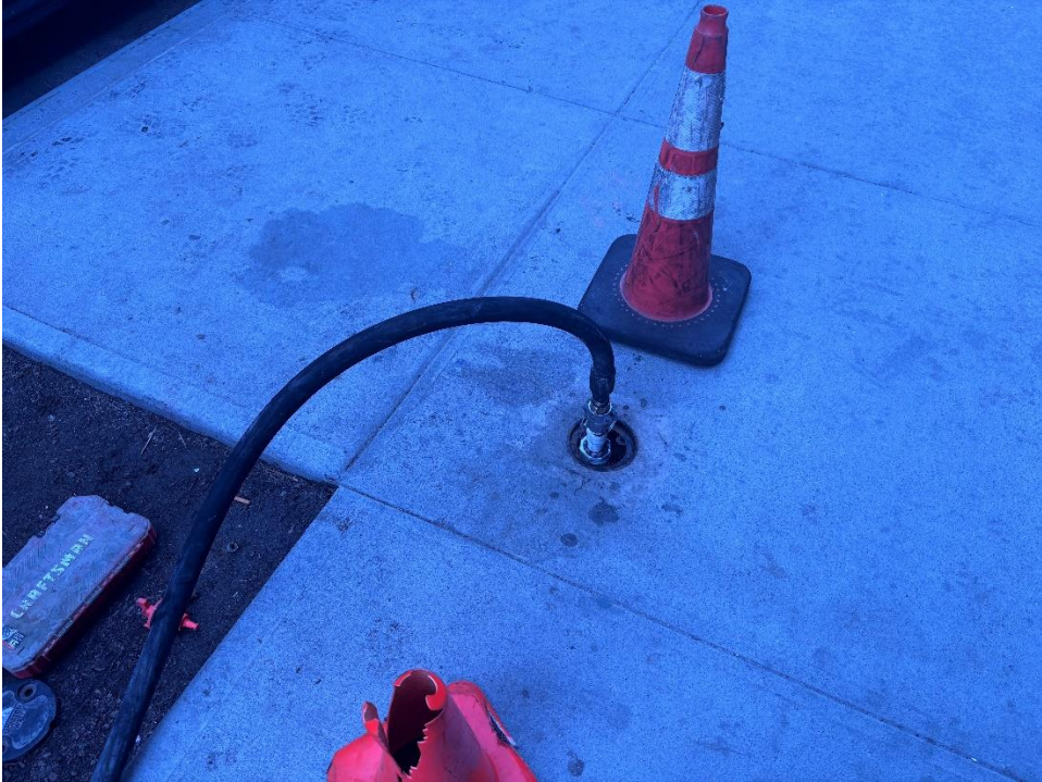
Photo 1: Injection housing and fittings connected to OMW-02
