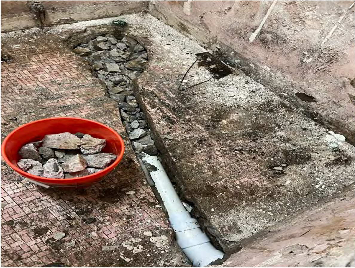
Existing concrete gouges that were sealed
