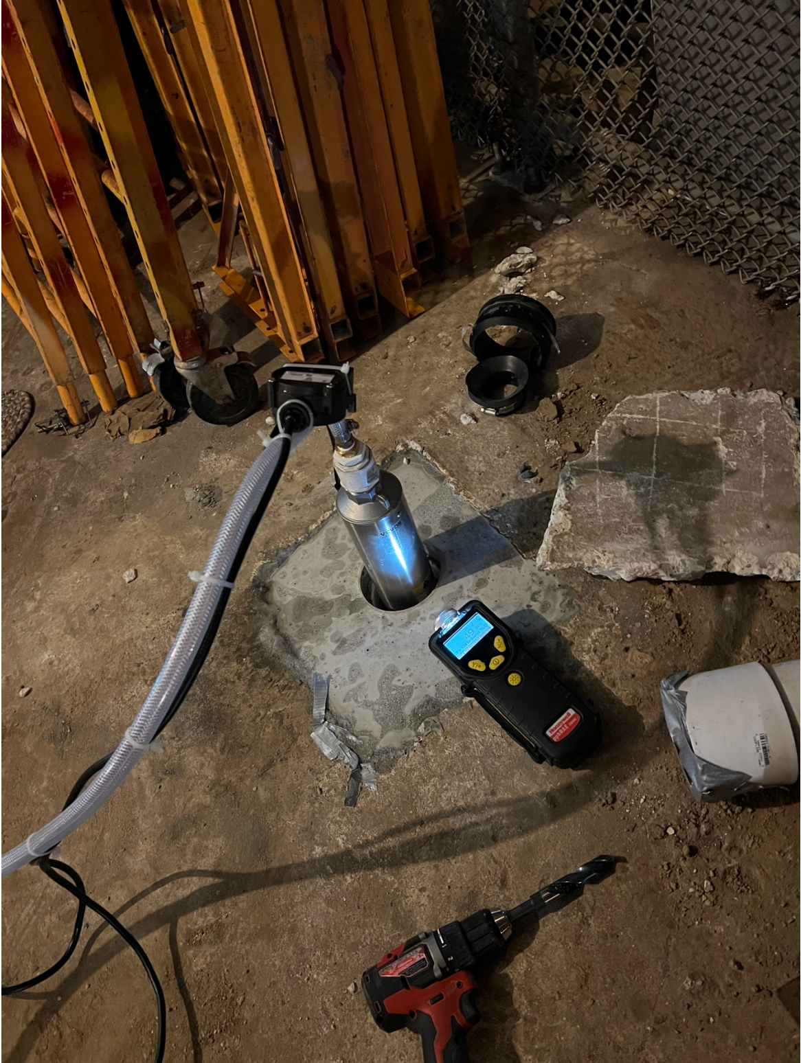
Dewatering Well with Pump
