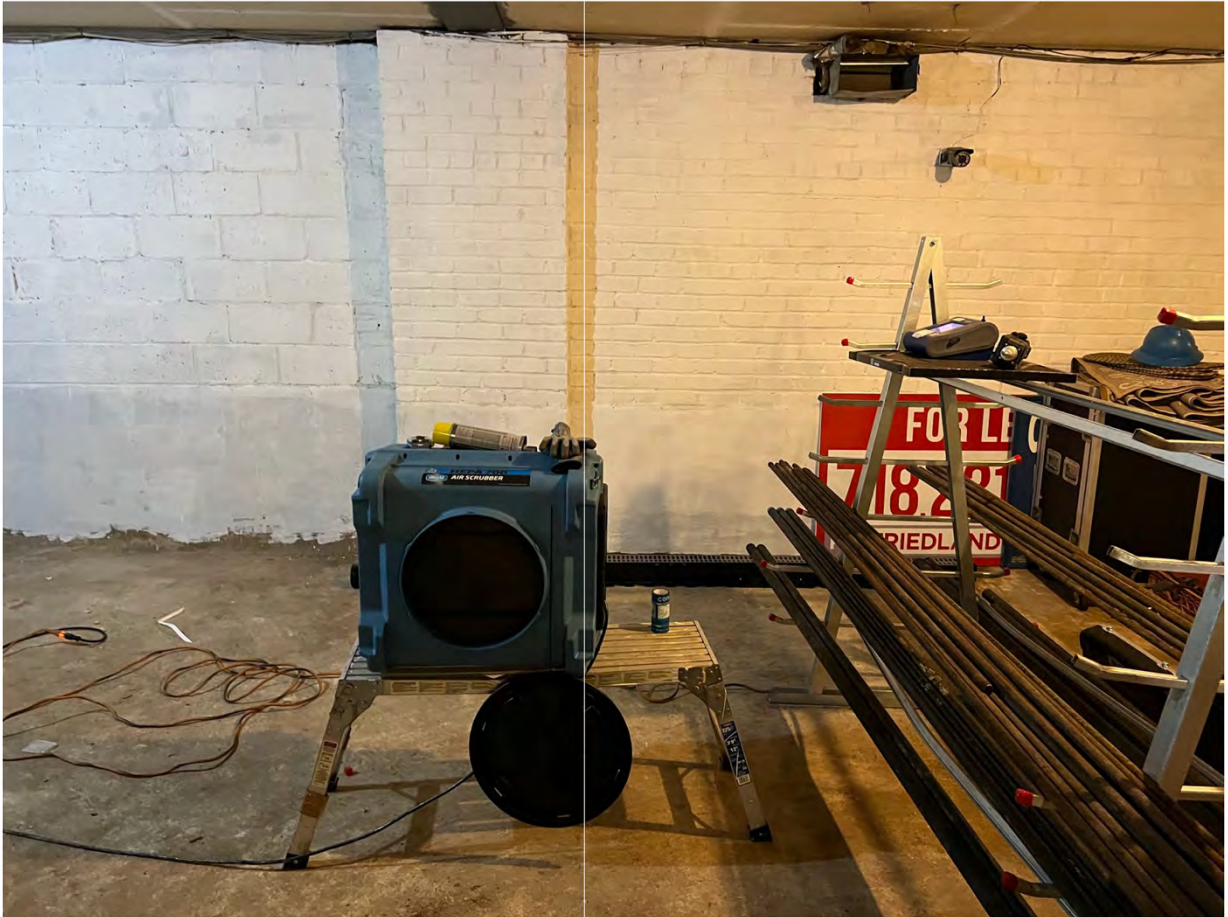
Dri-Eaz HEPA 700 Air Scrubber with an activated carbon filter
