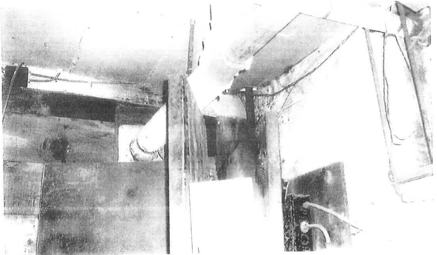
Pipes in basement
