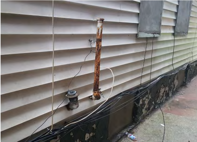
Vent & fill at 720 East 216th Street – front building
