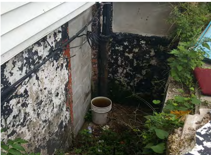
Sealed basement door
