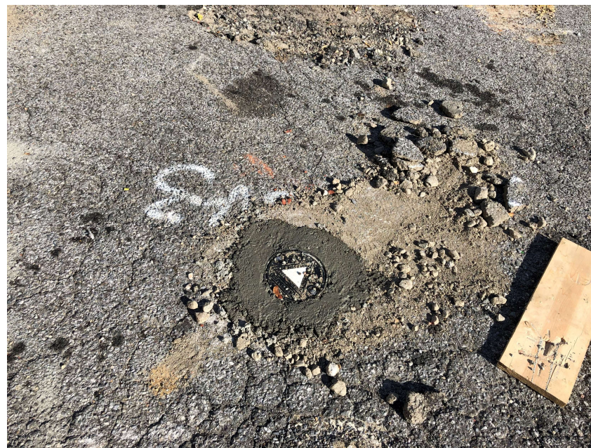
Soil Vapor Probe Secured with Manhole Cover
