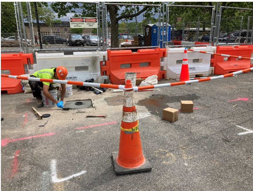
Photo 4: Looking south, view of AARCO finishing permanent well point MW-2 and SV-2.
