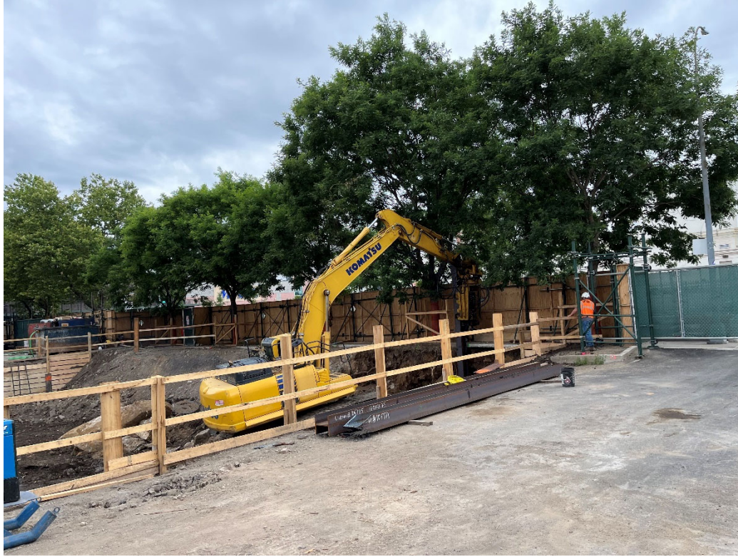
Photo 1: Looking northwest, Urban begins driving steel I-beams into the northern portion of the Site.
