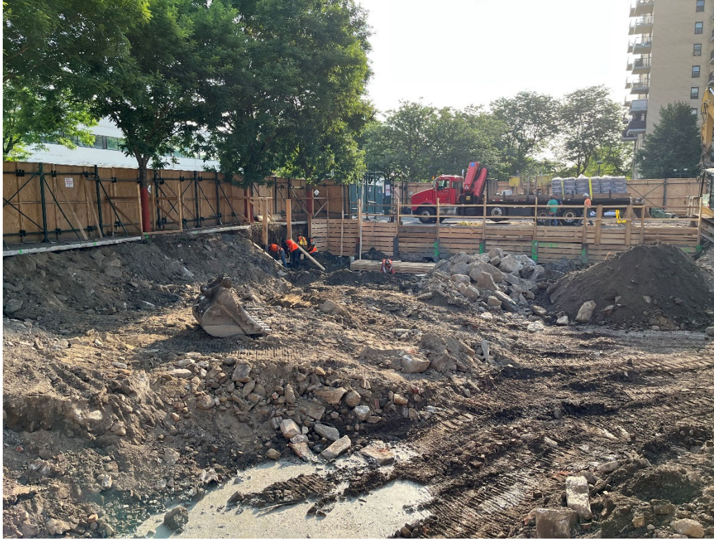
Photo 1: Looking northeast, Urban begins shoring along the northern edge of the Site.
