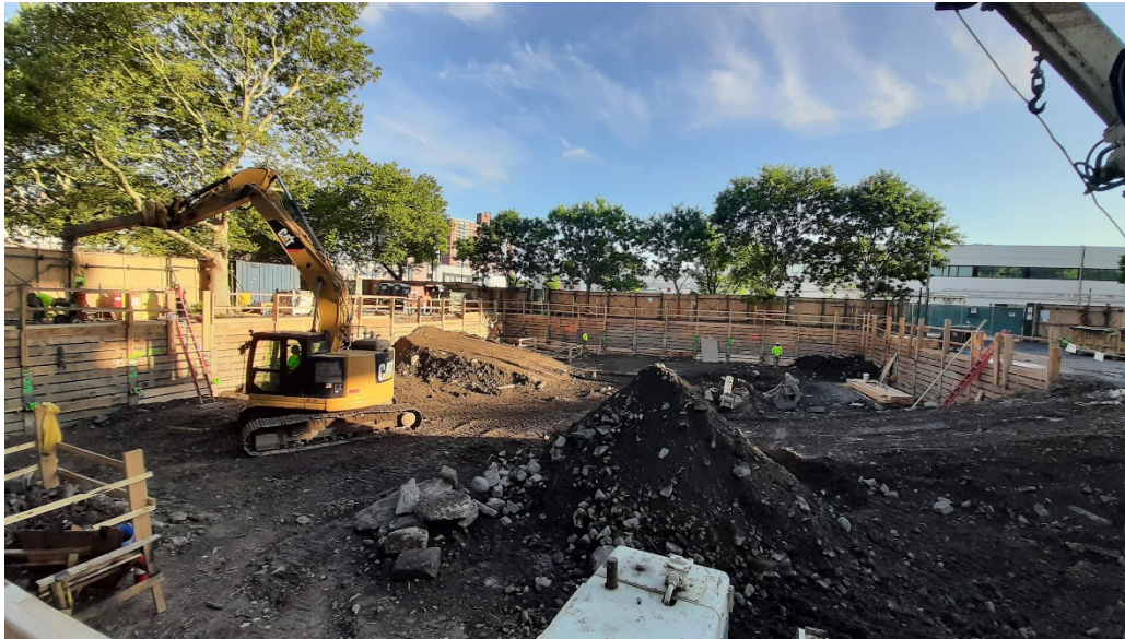
Photo 1: View facing N building footprint, morning progress of previous ramp (right) and the ramp's relocation (left).
