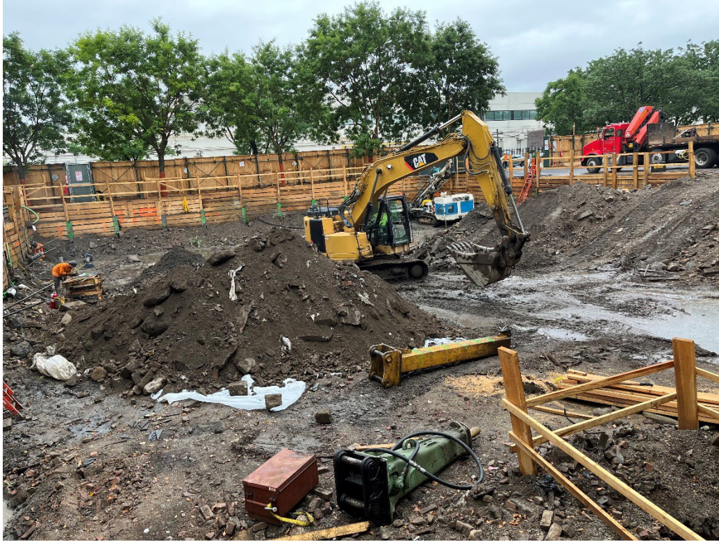
Photo 1: Looking north, Urban moves hazardous soil pile south to drive tie backs behind it.
