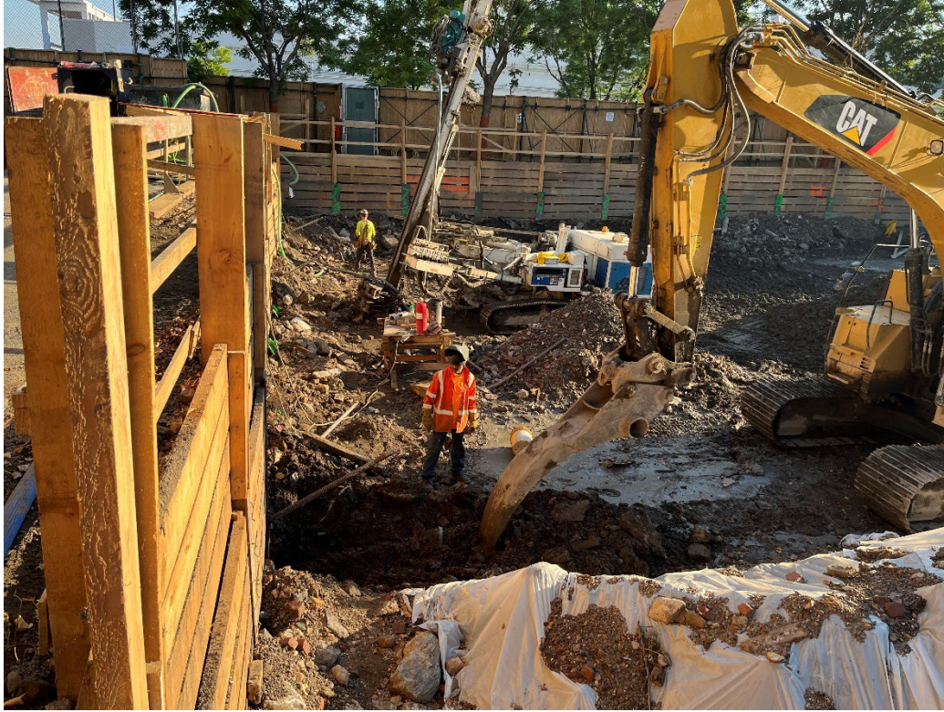
Photo 1: Looking north, Urban clears soil around tie backs to cut and prepare them.
