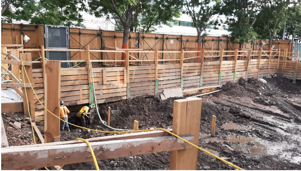
Photo 1: View facing N, work continues on shoring along the northern edge of excavation.
