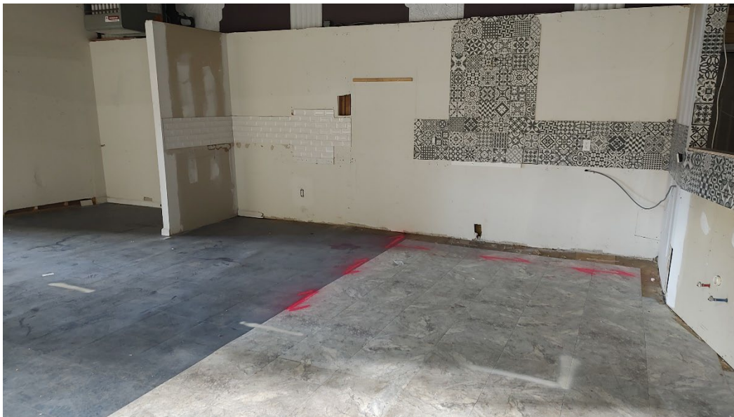
Photo 3 – View of the south end of the former kitchen warehouse with the partially detected unknown line.
