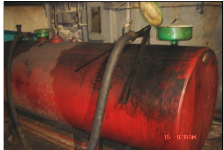
Photograph 12: Temporary AST in 1560 Boone boiler room.
