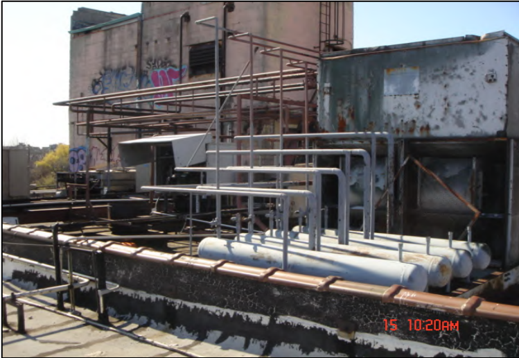
Photograph 17: Refrigeration equipment on 1560 Boone roof.
