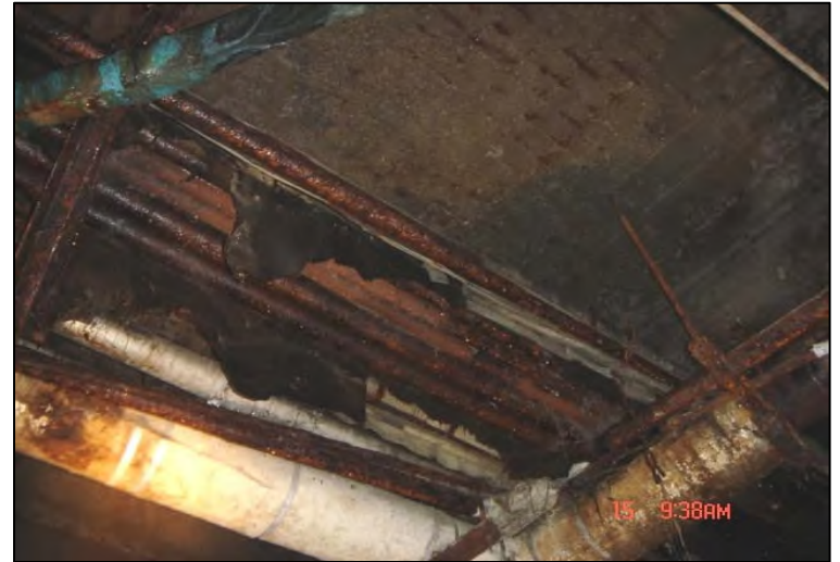
Photograph 14: PACM pipe insulation in "rock room".
