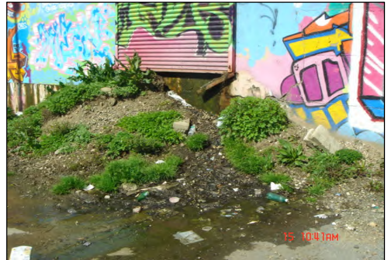
Photograph 6: Water seeping from the old tank room (rock room) along West Farms Road.
