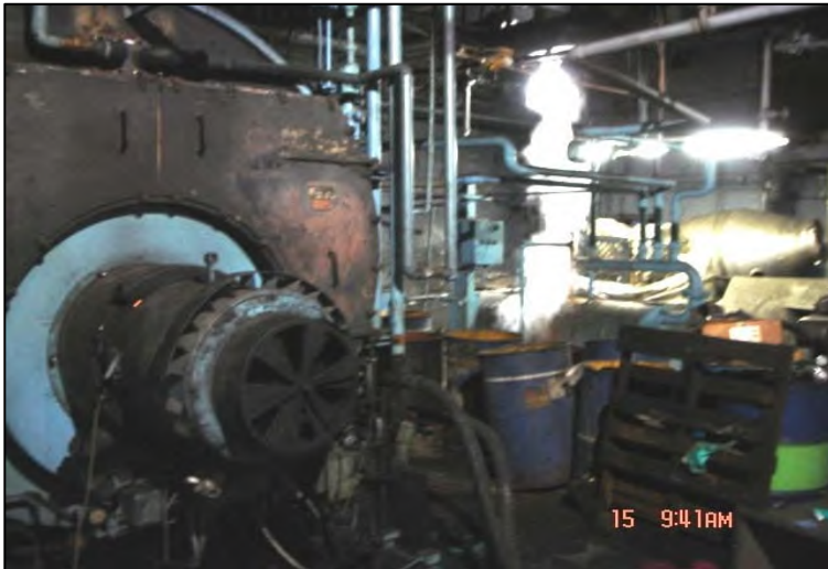
Photograph 13: Boiler room at 1560 Boone.
