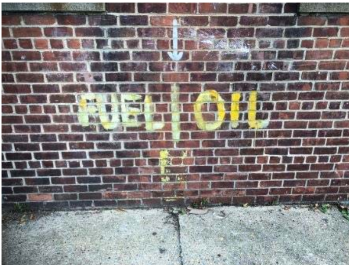
7. Former fill port associated with 2,500-gallon abandoned UST, located on western portion of building bordering Gerard Avenue.
