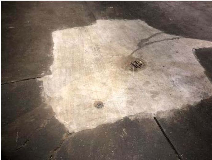
3. Floor drain and associated clean-out port.
