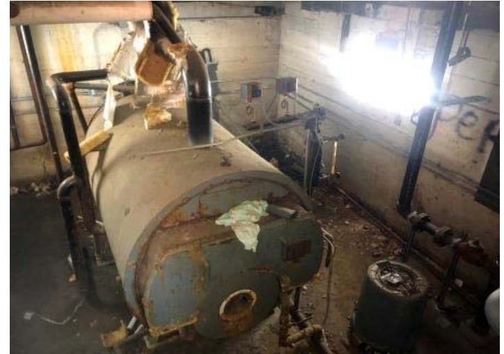
2. Sub-grade cellar and view of boiler.
