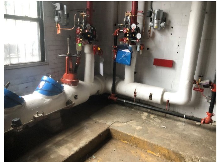
12. View of the fire department sprinkler system.
