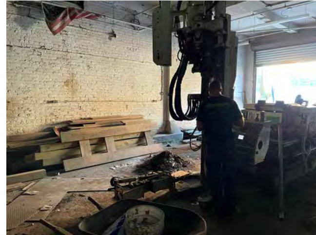
Photo 2: View of SB6/SV6 installation.
