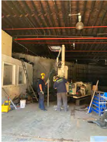
Photo 1: View of SB1/SV1 installation.
