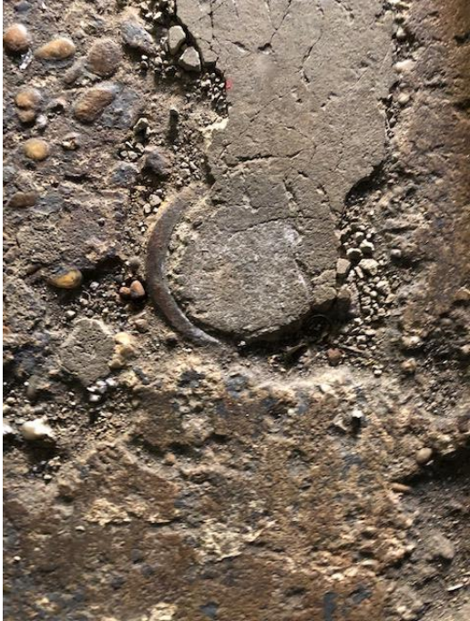
Pipe in the concrete floor – recommend investigation
