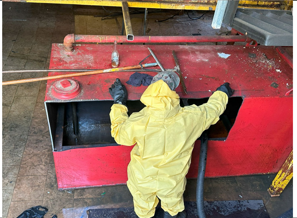
Photo 2: View of ABC tank vacuuming out the liquid contents of one of the 1,500 gallon AST.
