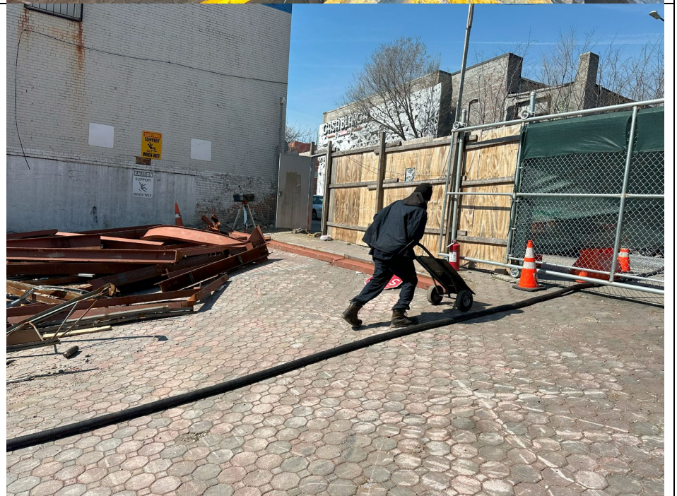
Photo 4: Worker from ABC removing disassembled portions of the empty and cleaned AST.
