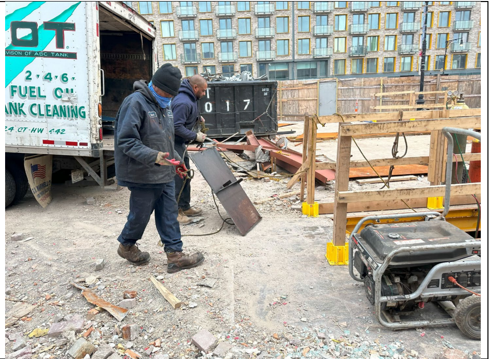
Photo 3: View of workers removing pieces of AST after welder disassembled the carcass.
