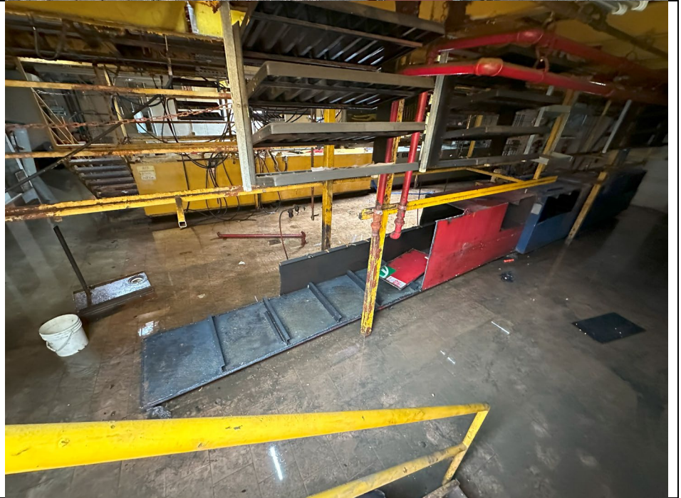
Photo 2: View of AST to be cut by welding, disassembled, and removed by ABC.
