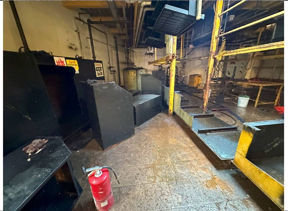
Photo 4: View of partially disassembled ASTs after work was completed for the day.
