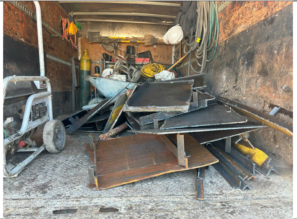
Photo 3: View of disassembled AST carcass pieces in the ABC truck for removal.
