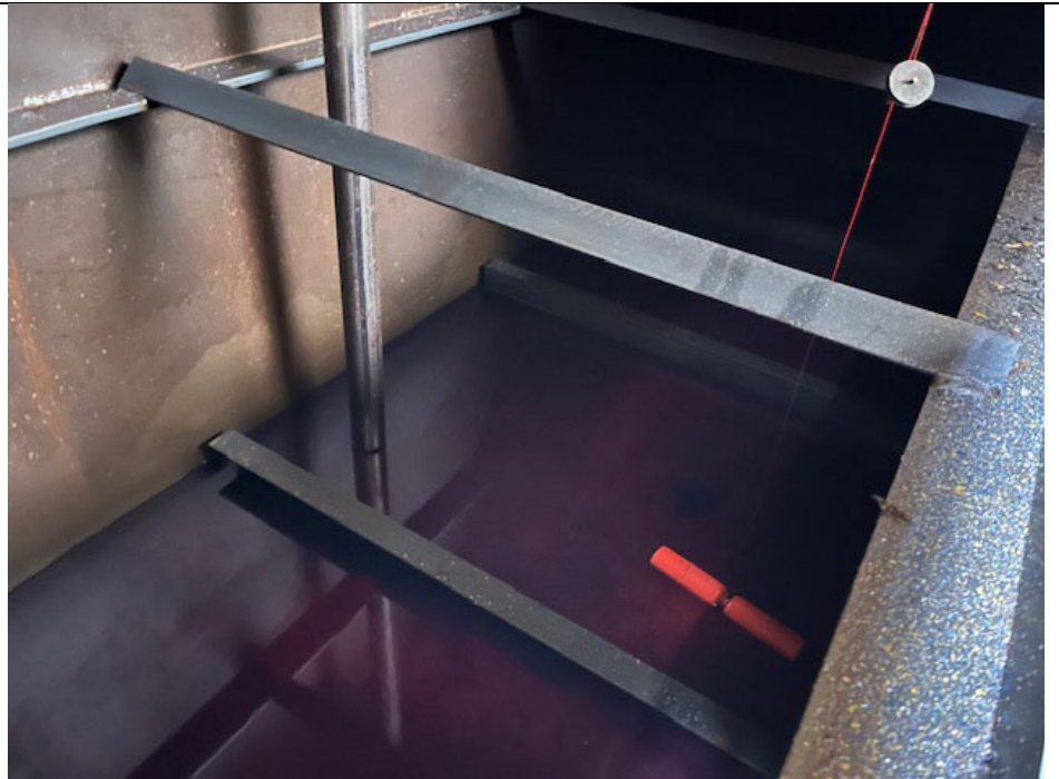
Photo 6: View of liquid contents in waste oil AST to be removed on 3/21/2024
