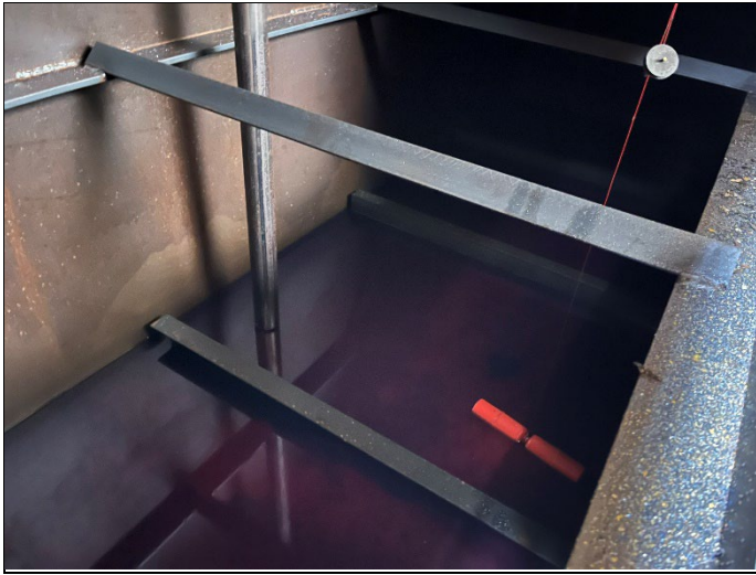
7. View of a few inches of liquid contents exposed
