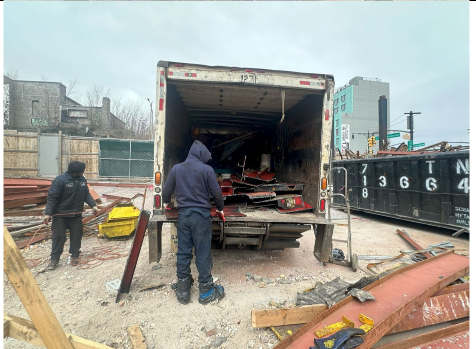
Photo 6: View of the ABC tank company truck at the end of the work day.
