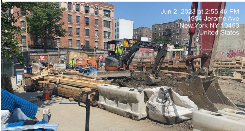
Photograph 3 - Light soil grading lasting roughly 10 minutes using only the small excavator. Facing East.
