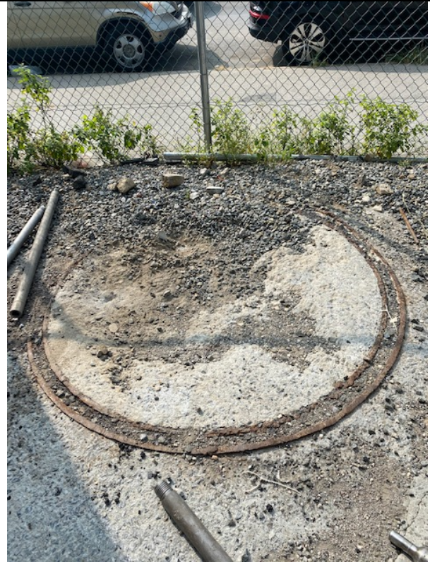
Suspect Manhole Cover at Subject Property
