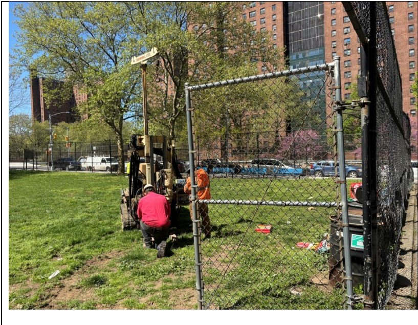
Photo 3: Looking south: View of GPI drilling soil boring for waste characterization sampling.
