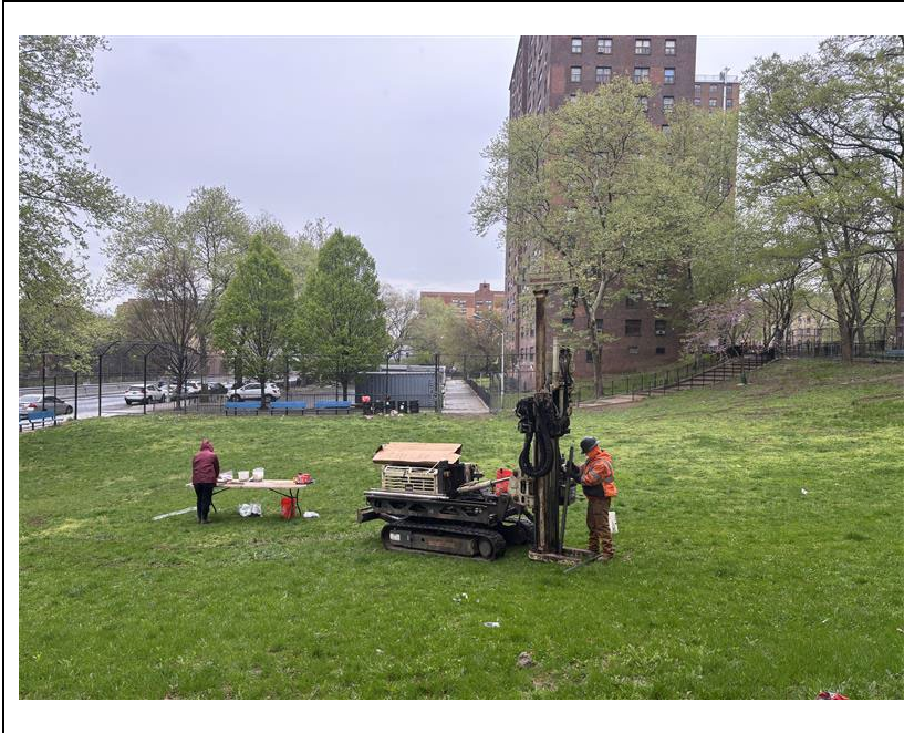
Photo 3: Looking north: View of GPI drilling soil boring for waste characterization sampling.
