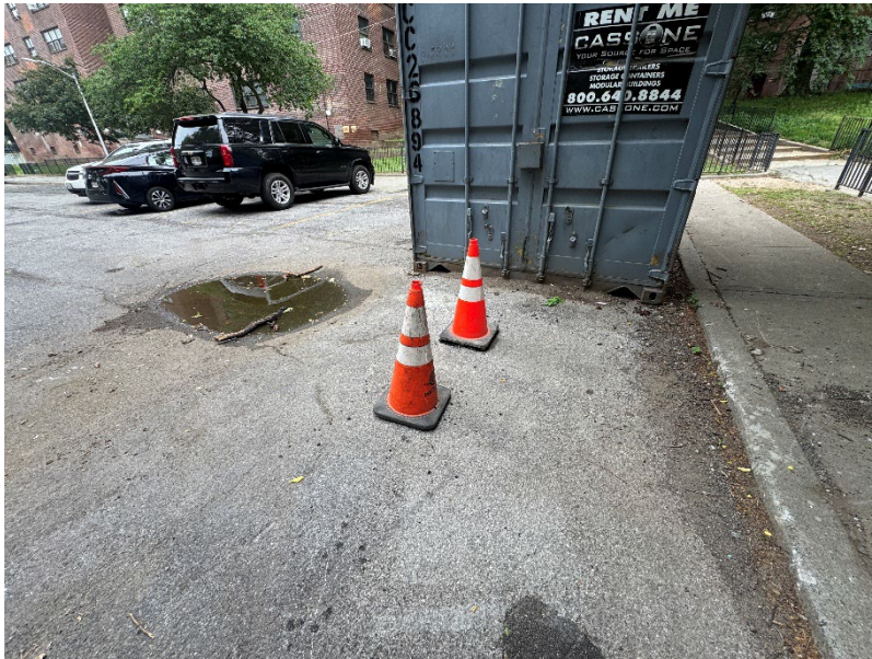
Photo 2: RIMW and RISV – 1 patched with asphalt and coned off.
