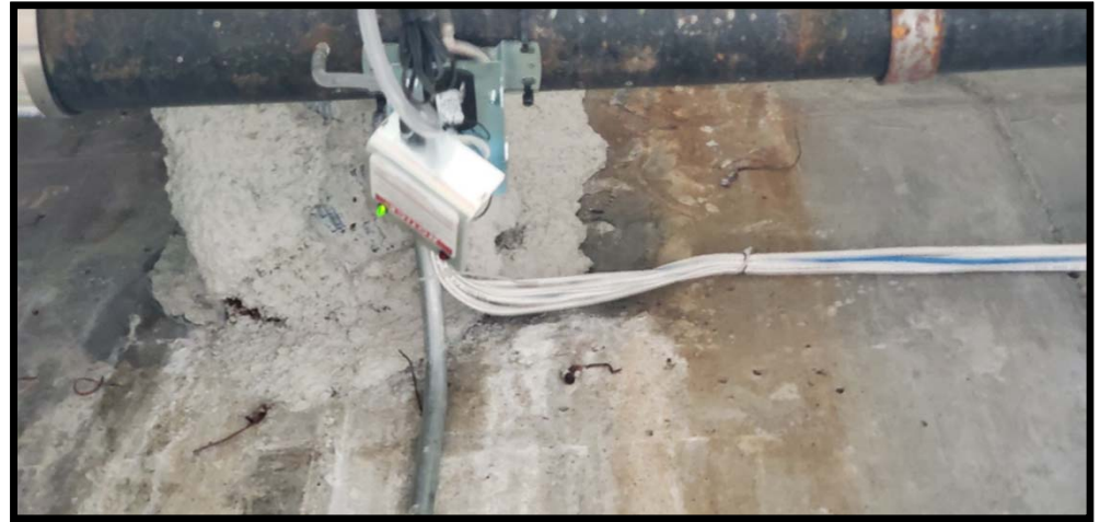
View of the alarm unit for the northern riser.
