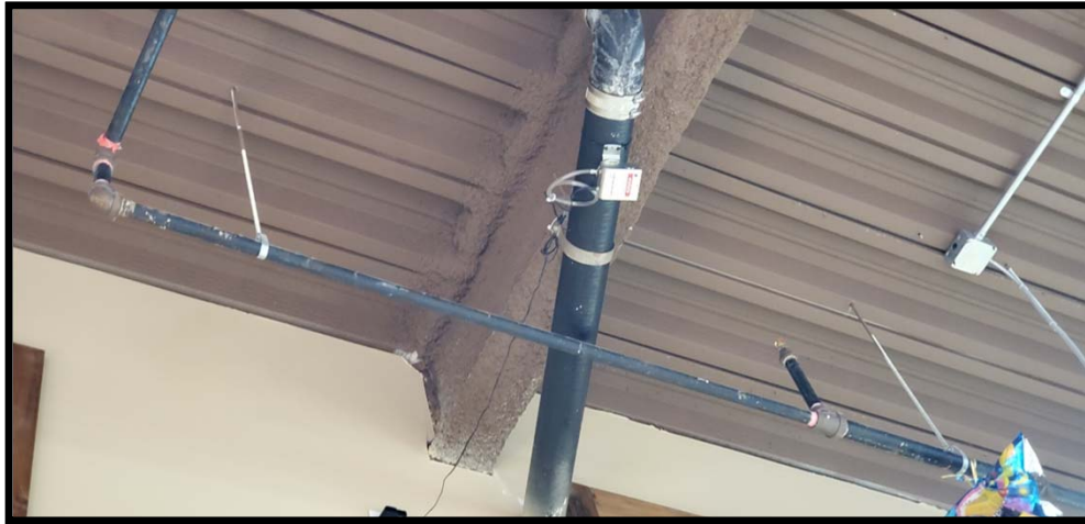
View of the alarm unit for the southern riser.
