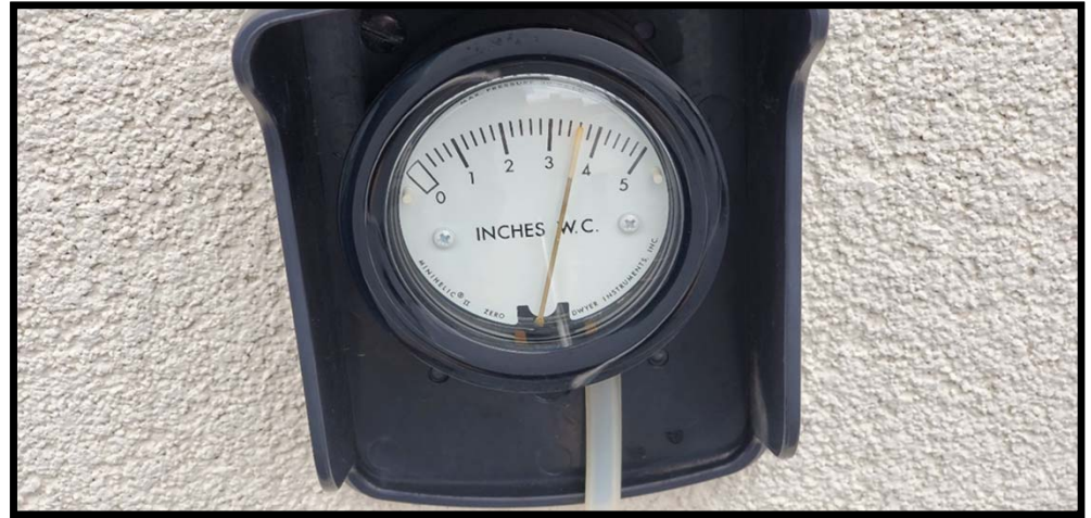
View of the gauge for the southern riser showing a vacuum pressure of -3.75 inches water column.
