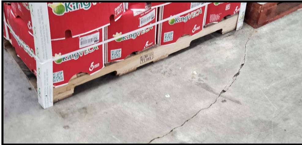
View of minor cracks in the basement floor. No vapor barrier is exposed.
