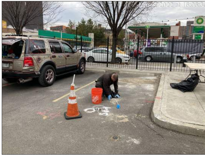
Photograph 5. Installation of temporary well and soil vapor point at location TW-04/SV-04 on the southern portion of the Site.
