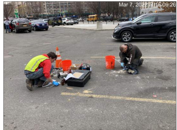
Photograph 8. Groundwater purging and sampling at location TW-01 on the western portion of the Site.
