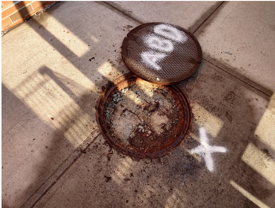
Photos 2 and 3 – One of two abandoned manholes on the property, filled with fill material.
