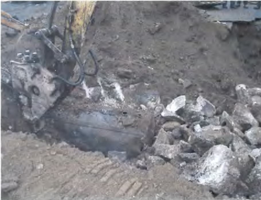
GASOLINE TANK UNCOVERED IN EXCAVATION
